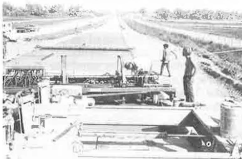
Figure 6. Form paver used on project I270 with machine used to insert plastic transverse weakened-plane joint and with bridge for burlap drag.
