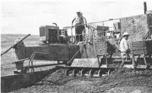
Figure 4. Paver used on project I80S with 15-kw, 180-cycle generator on right front leg of paver.
