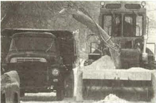
Figure 3. Snow blower mounted on the lift arms of an articulated wheel loader.
