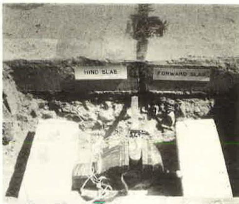
Figure 8. Test corners with low spot, with deflectometer pickup fixed under the hind slab 1 in. from center of expansion joint.
