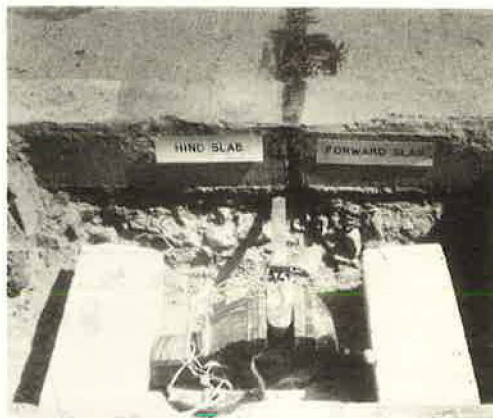
Figure 8. Test corners with low spot, with deflectometer pickup fixed under the hind slab 1 in. from center of expansion joint.
