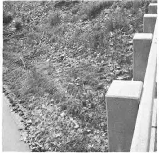
Figure 4. Condition of repaired area in 1969.
