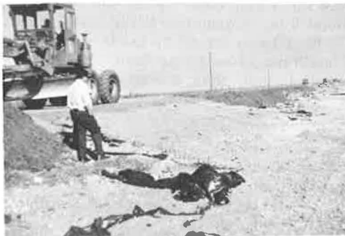
Figure 11. Condition of Louisiana Department of Highways test section after storm (in-place revetment underlaid with cloth Z).
