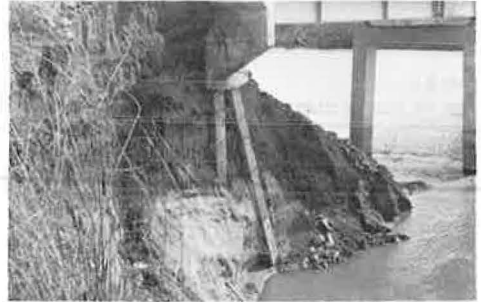
Figure 2. Conditions at bridge prior to repair work in 1962 by the Memphis District.
