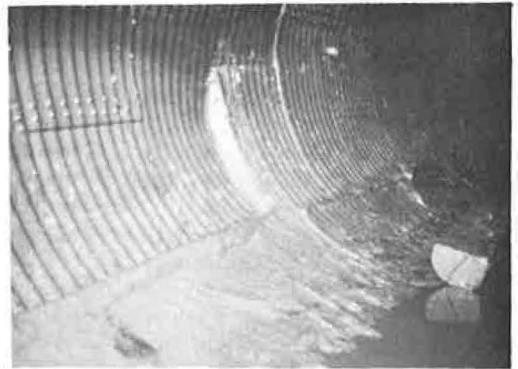
Figure 16. Failure of transverse joint in pipe shown in Figure 15.
