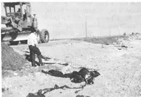
Figure 11. Condition of Louisiana Department of Highways test section after storm (in-place revetment underlaid with cloth Z).
