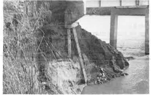
Figure 2. Conditions at bridge prior to repair work in 1962 by the Memphis District.
