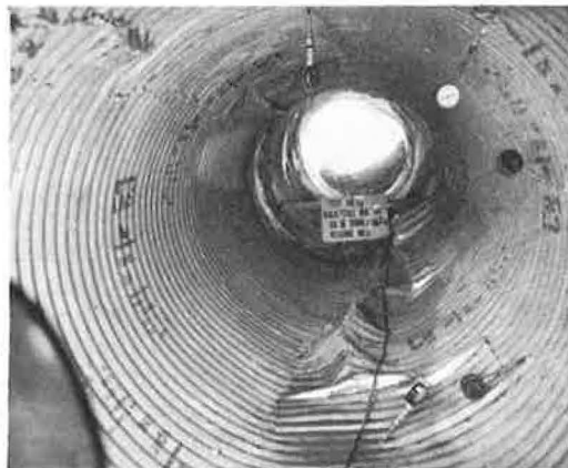
Figure 10. Pipe wall buckled at invert in dense soil (this is exceptional, for buckling is usually between 10 and 2 o'clock).
