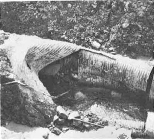
Figure 13. Complete collapse of 96-in. pipe.
