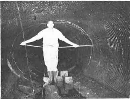
Figure 15. Excessive deflection of 84-in. storm sewer pipe.
