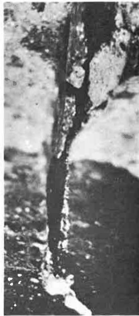
Figure 35. Damaged plane-of-weakness crack (unsealed joint).
