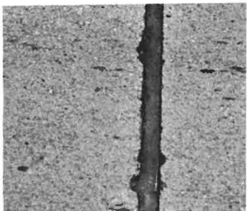
Figure 10. Coal-tar epoxy joint.
