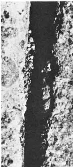
Figure 34. Close-up of core area (unsealed joint).
