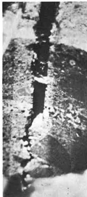
Figure 38. Plane-of-weakness crack (polysulfide-sealed joint).
