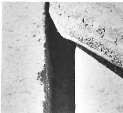
Figure 17. Clean joint with plane-of-weakness crack closed.
