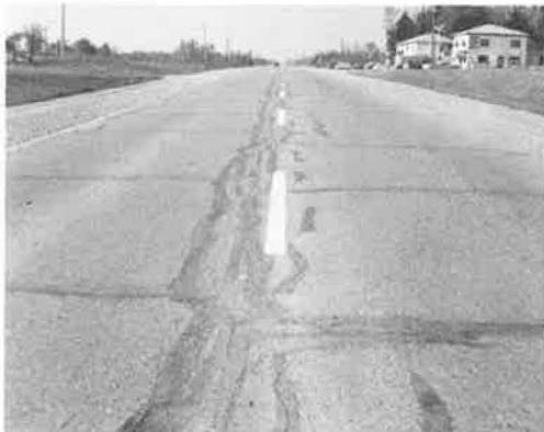
Figure 7. Transverse cracking (4-year old pavement made with 85- to 100-penetration asphalt).
