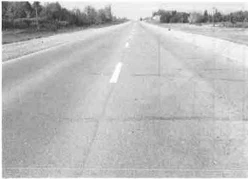
Figure 9. Transverse cracking (85- to 100-penetration asphalt, right lane).
