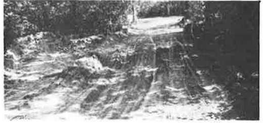
Figure 3. Poorly drained section in Virginia road.
