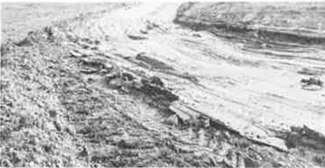
Figure 8. Deep depressions and potholes in Mississippi road.
