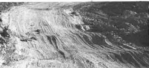
Figure 10. Deep depression, washboarding, and soil buildup in SEA road.
