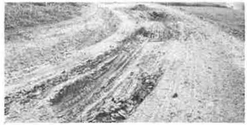
Figure 7. Deep potholes in Mississippi road.
