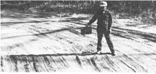
Figure 2. Potholes in Virginia road.
