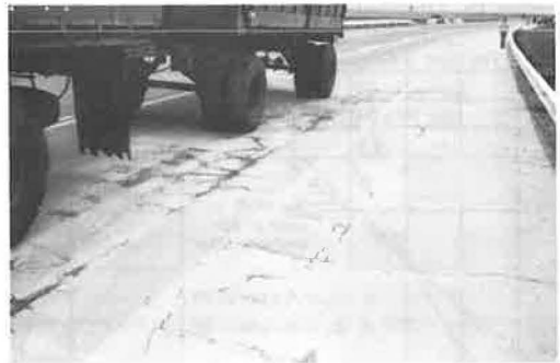
Figure 20. Overall view of pavement showing typical crack pattern.
