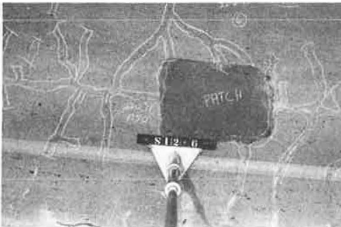
Figure 19. Crack pattern, February 22, 1971.
