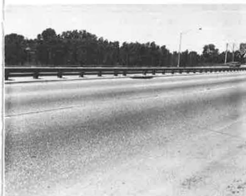
Figure 5. Wheelpath wear on asphaltic concrete with gravel aggregate.
