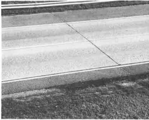
Figure 1. Wheelpath wear on PCC pavement with gravel aggregate.
