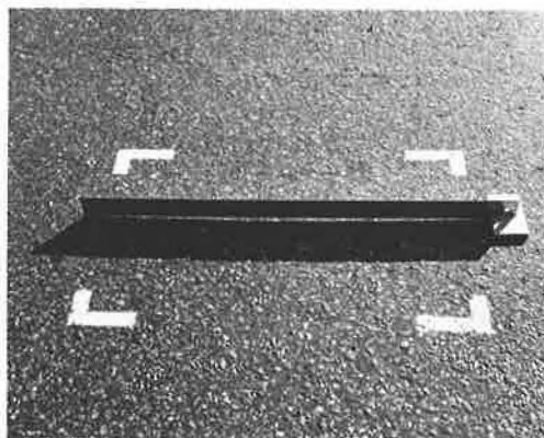
Figure 6. Depth of wheelpath wear on asphaltic concrete.
