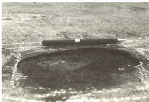
Figure 6. Example of 1/4- to 1/2-in. deep spall.
