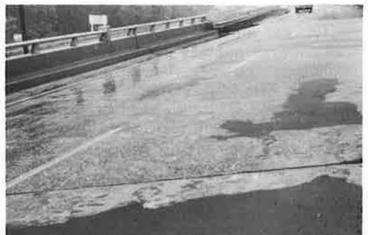
Figure 12. Site of several skidding accidents on downhill, superelevated deck treated with epoxy surface treatment with no initial deslicking sand applied.
