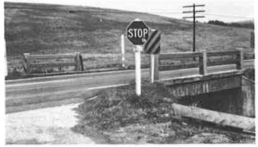
Figure 3. Same bridge shown in Figure 2 with east end of north rail knocked out.
