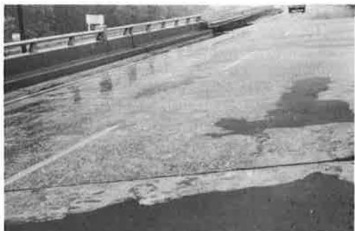
Figure 12. Site of several skidding accidents on downhill, superelevated deck treated with epoxy surface treatment with no initial deslicking sand applied.
