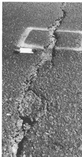
Figure 5. Wide transverse crack in asphalt pavement over contraction joint in reinforced concrete base (section G).
