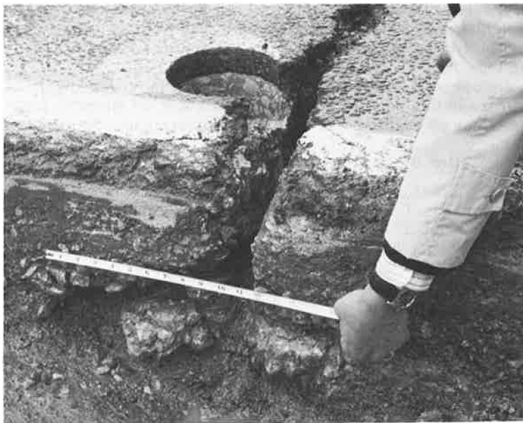
Figure 7. Severe spalling in bottom half of concrete base slab at wide crack (section D).
