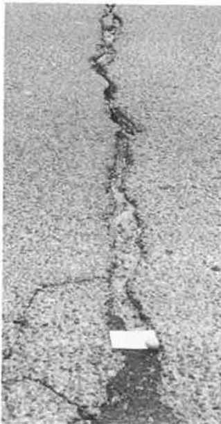
Figure 4. Wide transverse crack in asphalt pavement on unreinforced concrete base (section A).
