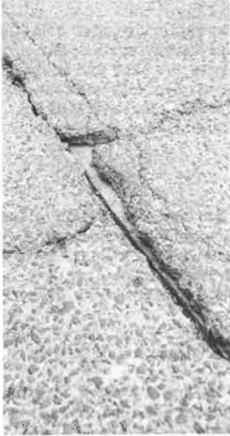
Figure 9. Loss of asphalt pavement due to cracking at centerline joint (section D).
