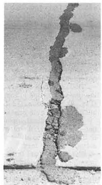
Figure 6. Wide stepped transverse crack, about 3 1/2 in. wide, in continuously reinforced concrete pavement (section H).
