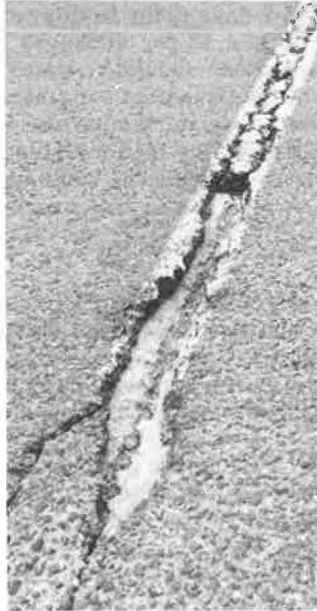
Figure 10. Loss of asphalt pavement due to cracking at centerline joint (section F).
