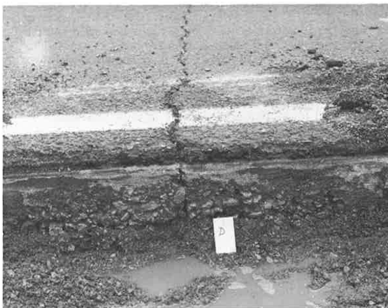
Figure 8. Less severe spalling near base of concrete slab at narrow crack (section D).
