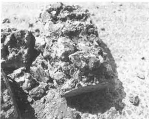
Figure 12. Breakdown of macadam mix binder course due to stripping of asphalt film from coarse aggregate particles (section B).
