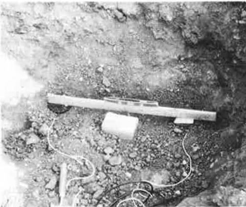
Figure 9. Sensors and remote readout settlement platform in position during checking of level of plane of sensors.
