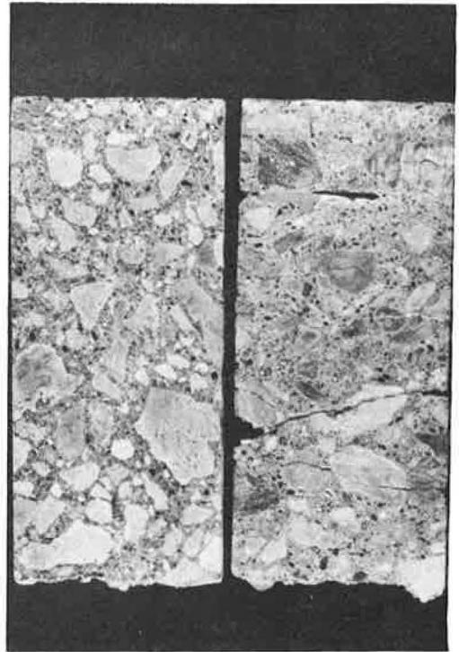
Figure 3. Vertical sections of cores taken on each side of transverse joint shown in Figure 2.
