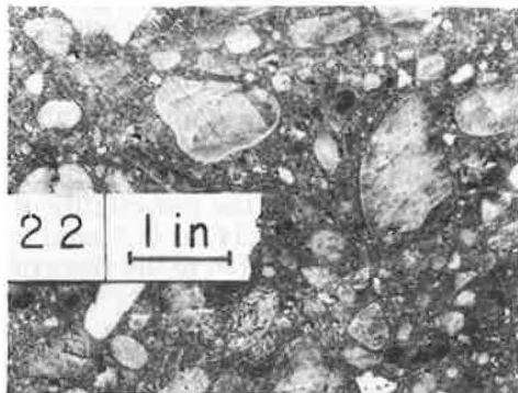
Figure 1. Concrete made with traditional sand and gravel according to curve 1 shown in Figure 2 (6).
