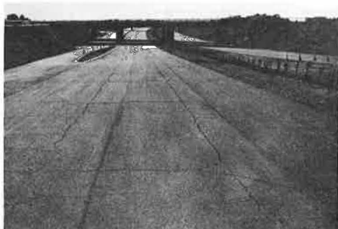
Figure 1. Pavement showing block cracking of lean-mix concrete base.
