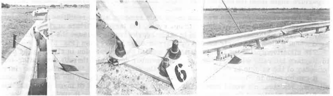
Figure 5. Damage to MBGF.
