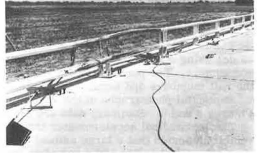
Figure 7. Damage to E-3 barrier.
