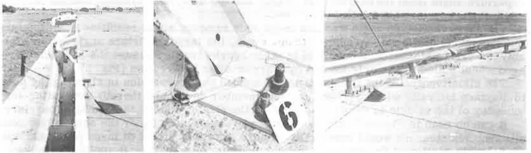
Figure 5. Damage to MBGF.
