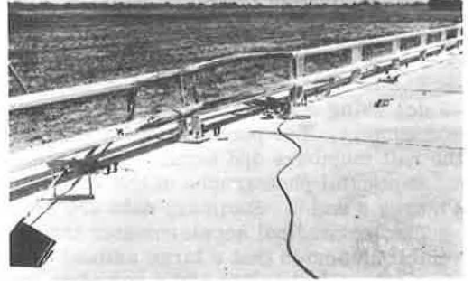
Figure 7. Damage to E-3 barrier.
