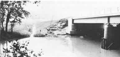
Figure 10. Upstream view of scoured bridge abutment and approximately 2 ft of exposed piling on Canisteo River bridge.
