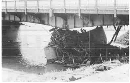
Figure 13. Settlement due to scour on Chemung River bridge in Elmira, N.Y.
