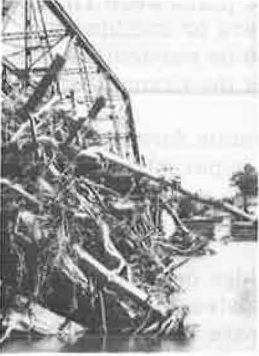
Figure 1. Debris deposited on bridge by floodwaters.
