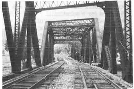
Figure 20. Downstream view of Lehigh Valley Railroad bridge showing pier settlement.
