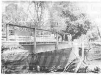
Figure 2. Cracked pier cap on Towanda Creek bridge in Powell, Penn.
