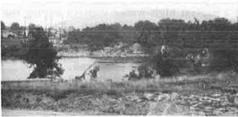
Figure 19. Upstream scour hole, eroded approach embankment, and damaged abutment of Lehigh Valley Railroad bridge.
