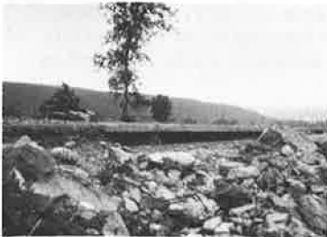
Figure 22. Undermined roadway slab and scoured embankment fill adjacent to Tioga River.
