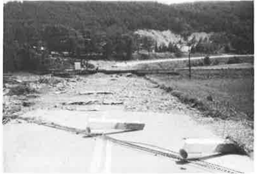
Figure 8. Approach damaged by overflow on Tioga River bridge.
