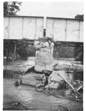
Figure 24. Front view of cracked pier shaft and broken pier footing.
