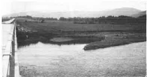
Figure 17. Enlarged scour hole upstream from Chemung River bridge in Waverly, N.Y.
