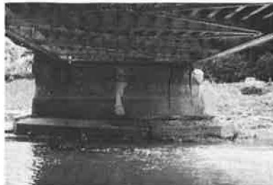
Figure 23. Cracked pier shaft supporting a county bridge on Schrader Branch of Towanda Creek.
