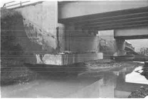
Figure 12. Scour beneath and behind abutments on US-15 interchange bridge.
