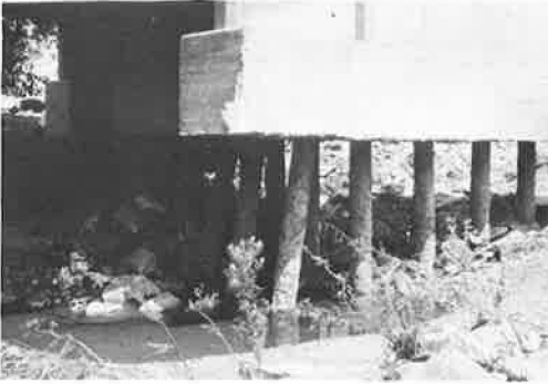
Figure 7. Approximately 7 ft of exposed piling beneath abutment of Tioga River bridge.
