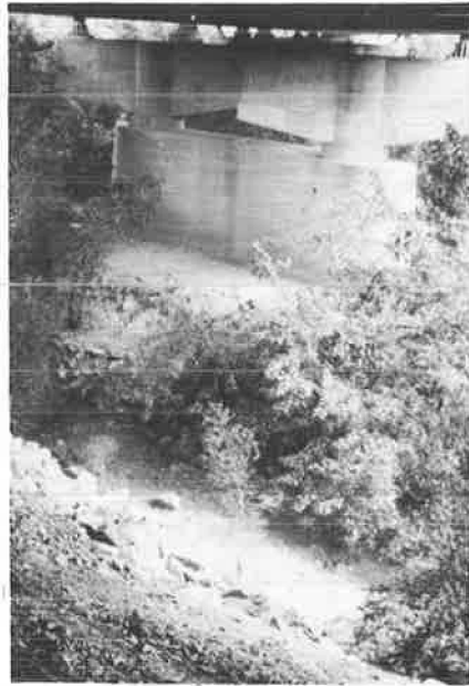
Figure 15. Post-flood condition of floodplain between abutment and adjacent pier of Susquehanna bridge.
