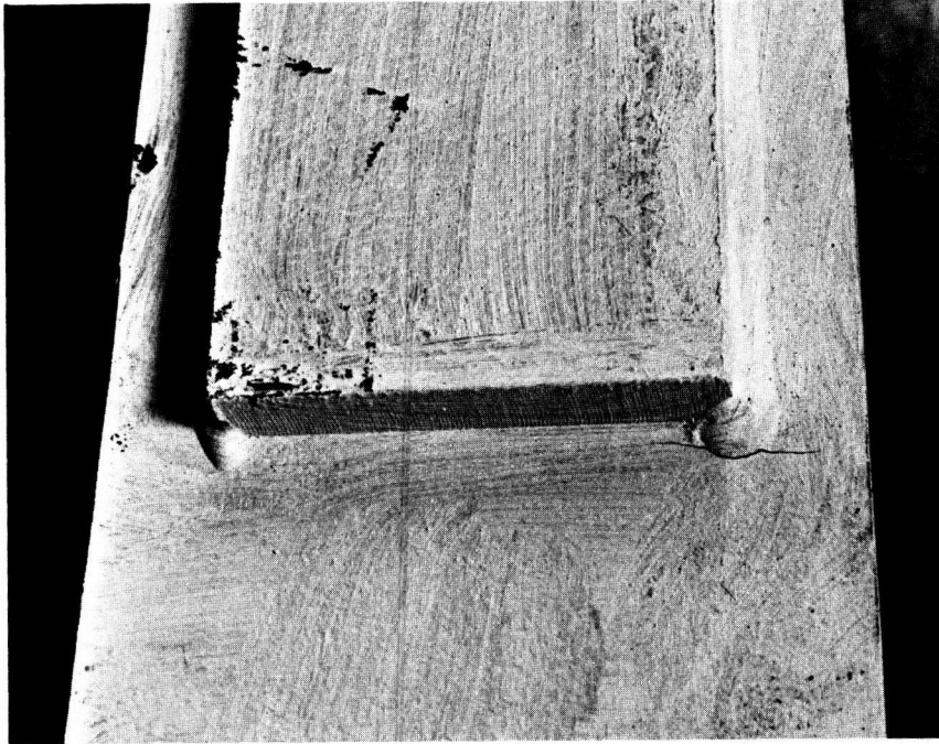
Figure 11. Crack formation at toe of longitudinal fillet weld.
