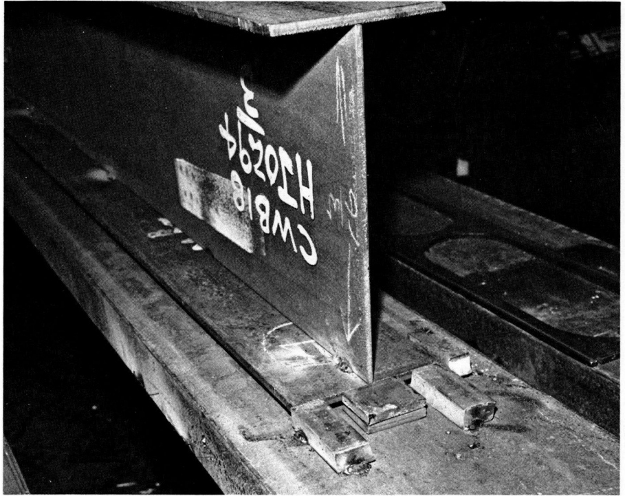
Figure C-3. Tack welds along web-flange junction.
