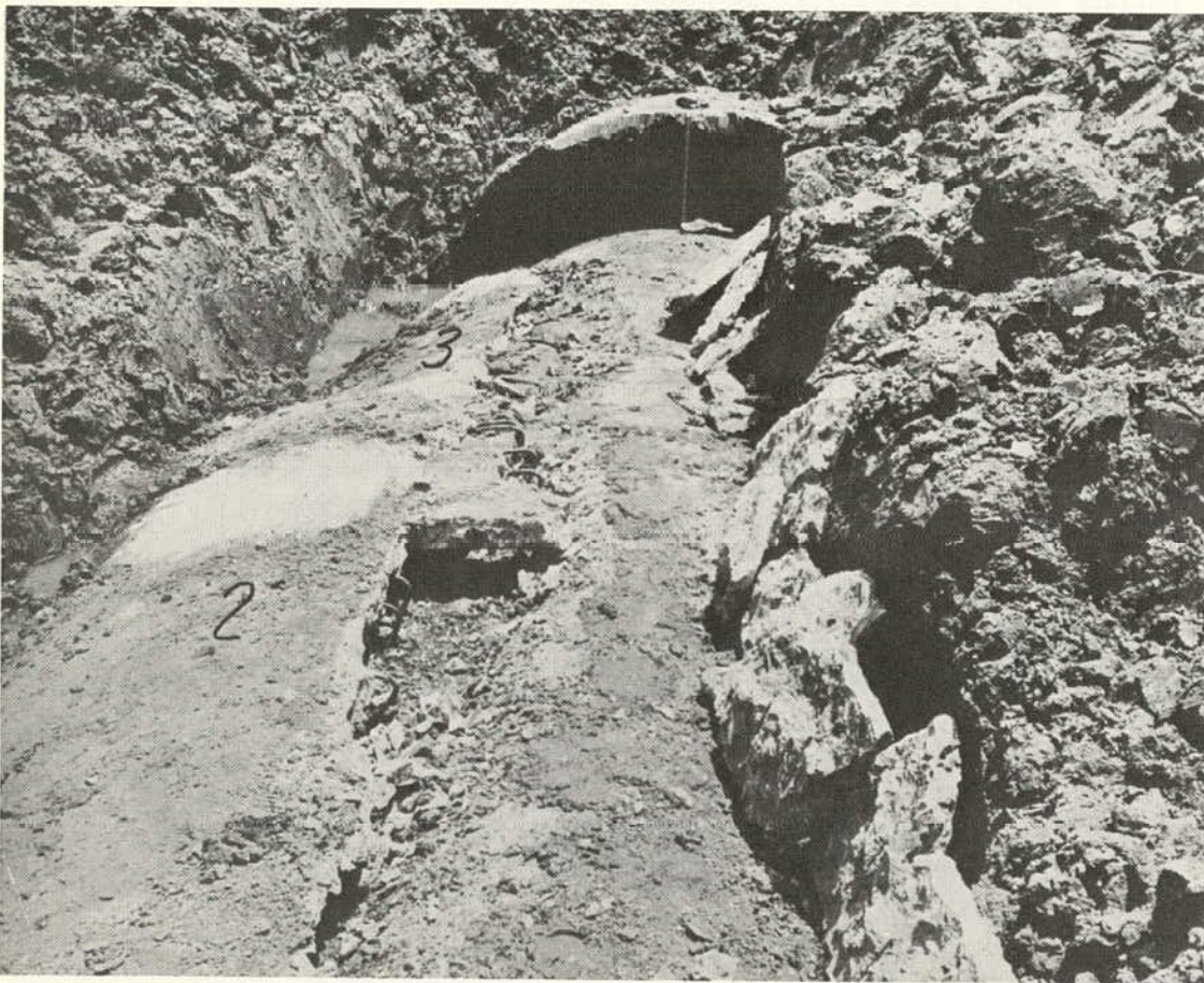
Figure J-9. Top of pipe after failure (Case 9).
