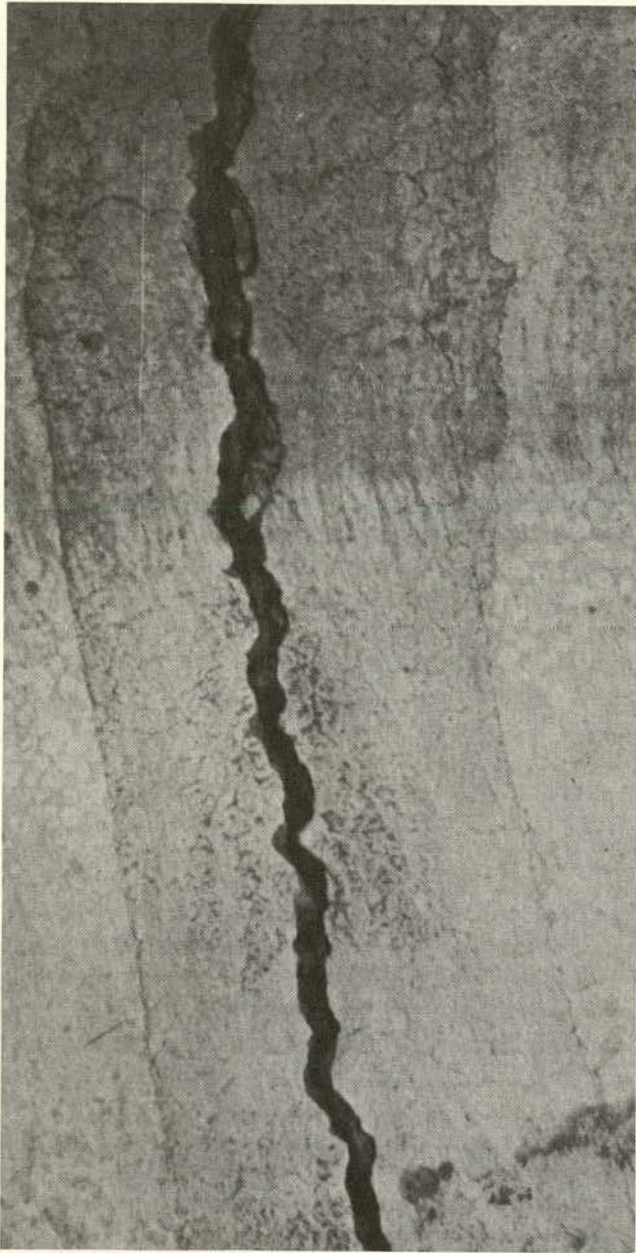
Figure J-7. Circumferential break in reinforced concrete pipe (Case 7). This crack was \frac{3}{8} to \frac{3}{4} in. wide at the crown and \frac{1}{8} to \frac{1}{4} in. wide at the invert.
