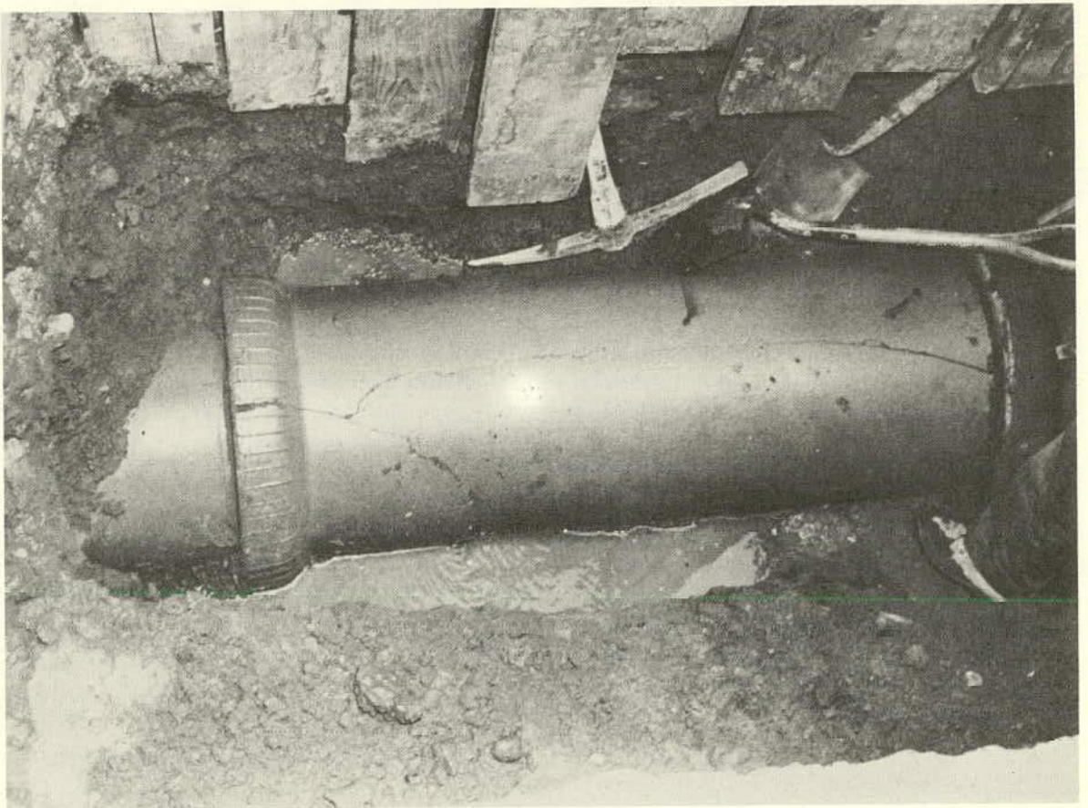
Figure J-12. Broken 18-in. clay pipe (Case 10).
