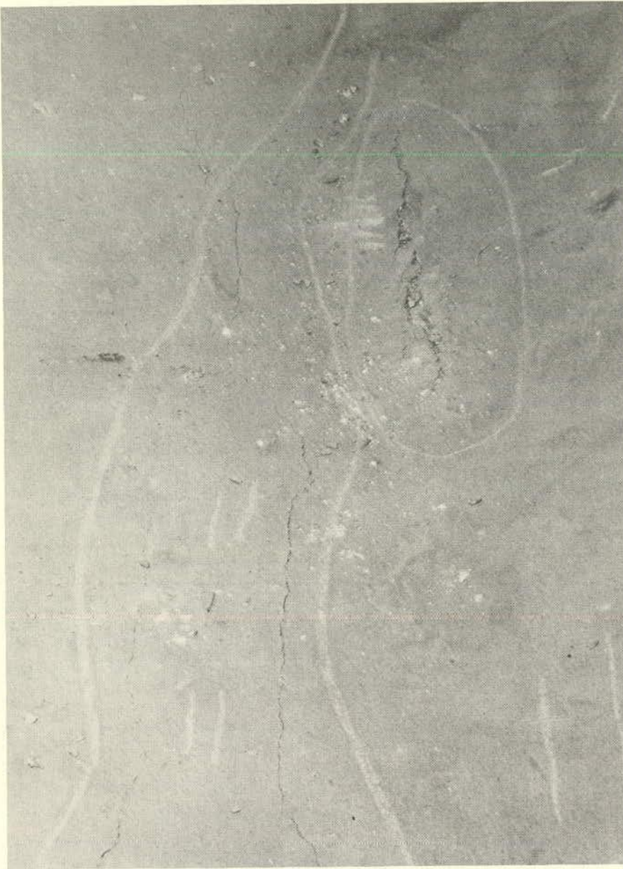
Figure J-3. Longitudinal cracks and spalled concrete in invert (Case 2).
