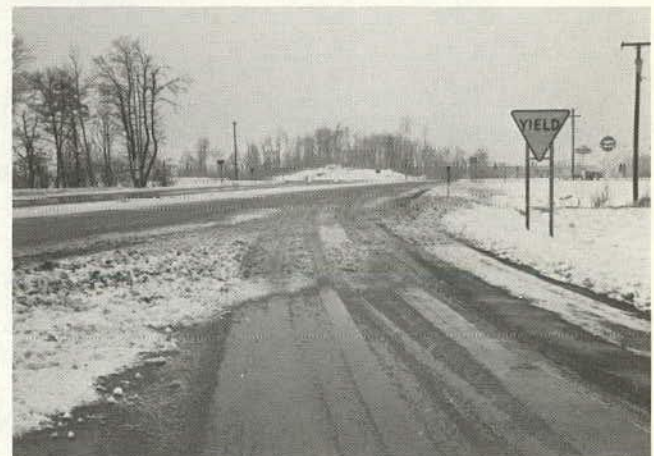
Figure 12. Windrows deposited across ramp openings.
