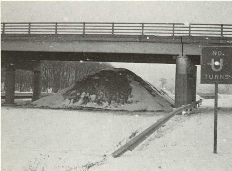
MATERIAL STORAGE UNDER STRUCTURE
