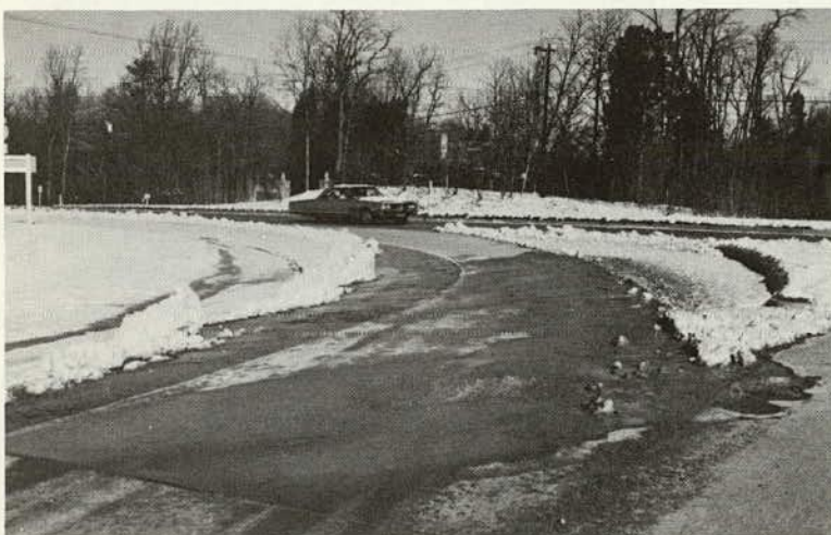
Figure 13. Melt water flowing across superelevated ramps.
