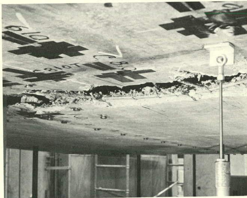
Fig. D-69 Region of Initial Spalling after Test to Destruction of Double-Column Model Bridge
