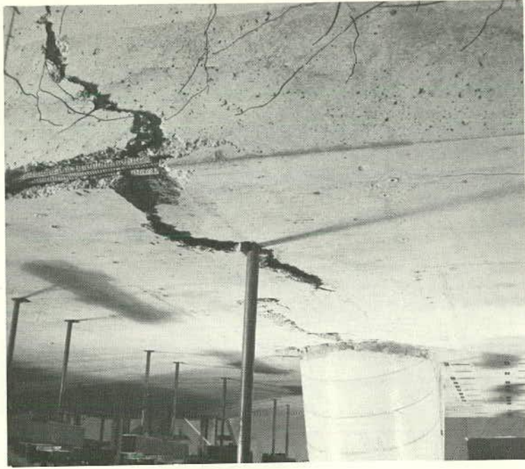
Fig. E-44 Crushed Concrete of Specimen SF-4
