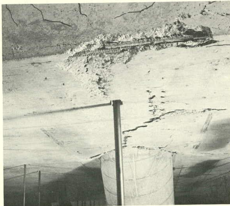
Fig. E-50 Crushed Concrete of Specimen SF-5
