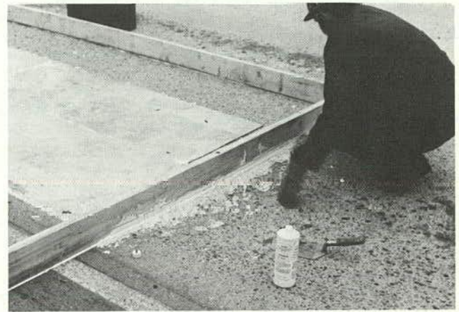
Figure H-24. Sealing dike (note prior sealing of area already dried at left).
