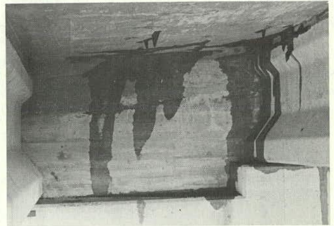
Figure H-10. Monomer leakage from underneath slab at free edge.
