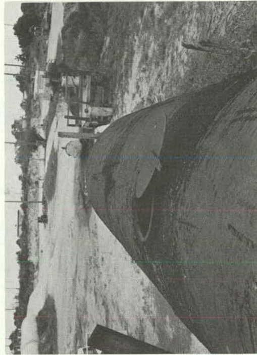
Figure F-7. Hubbard Construction Co. RC-70 storage tank hatch open for sampling.
