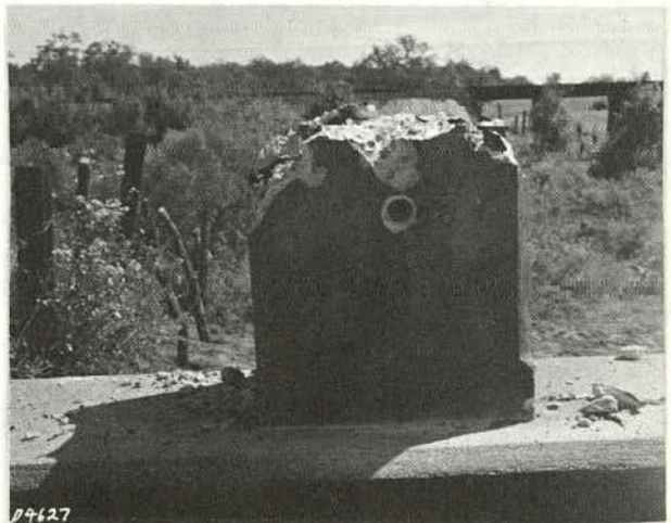
Figure 12. Picture shows how a tamp-in was placed in this existing concrete post so that the flex-beam rail could be attached.
