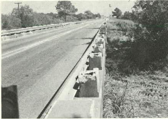
Figure 13. Flex-beam rail attached to concrete posts.
