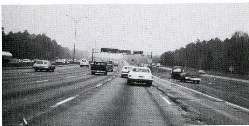
Figure 21. Acceptable conversion of right shoulder to full running lane because of ample flat graded area between freeway and frontage road (note pavement deterioration at old shoulder - main-lane joint).
