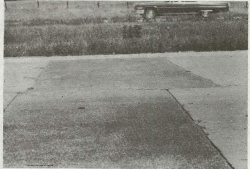
Figure 82. Low-Severity Asphalt Patch Deterioration.
