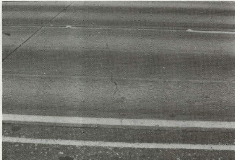
Figure 52. Low-Severity Transverse Crack.
