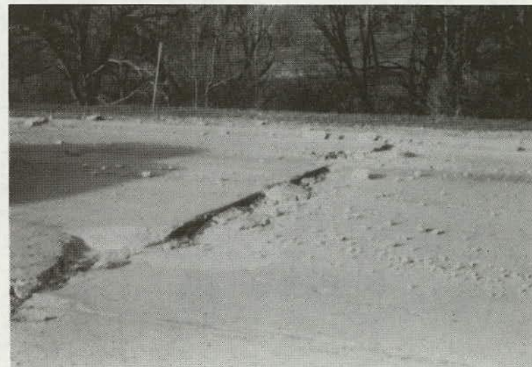
Figure 58. High-Severity Shattering Type Blow-up.
