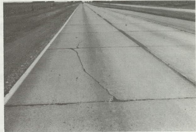
Figure 27. Medium-Severity Longitudinal Crack.
