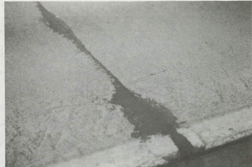
Figure 69. Low-Severity Joint Seal Damage.
