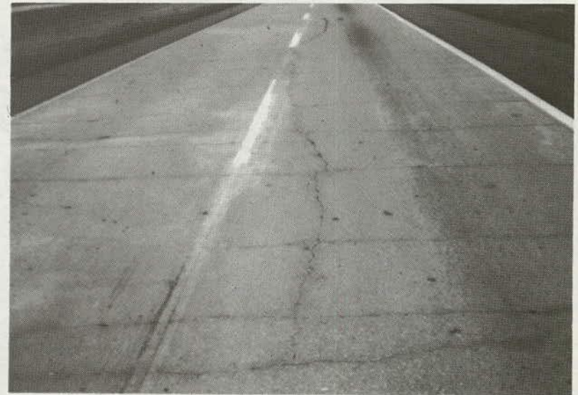
Figure 131. Medium-Severity Longitudinal Crack.
