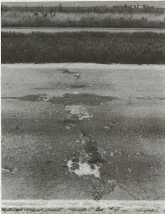
Figure 65. High-Severity "D" Cracking.
