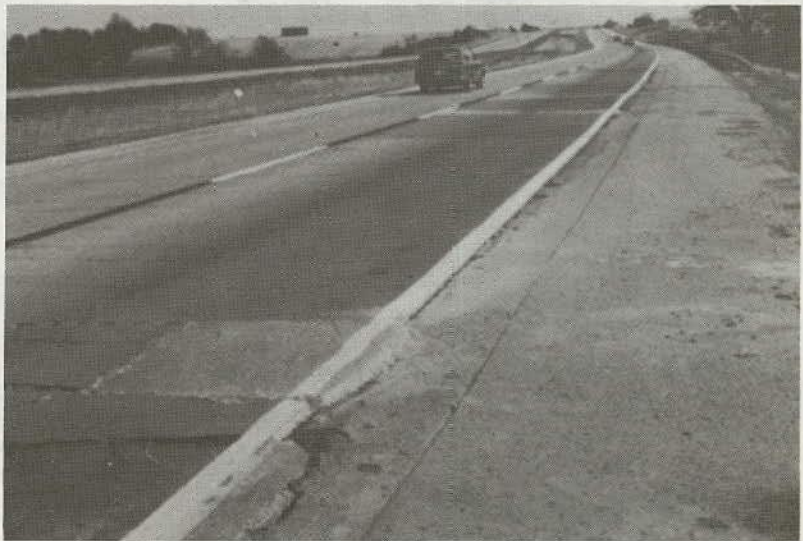
Figure 149. Very-High-Severity Pumping of Fines.
