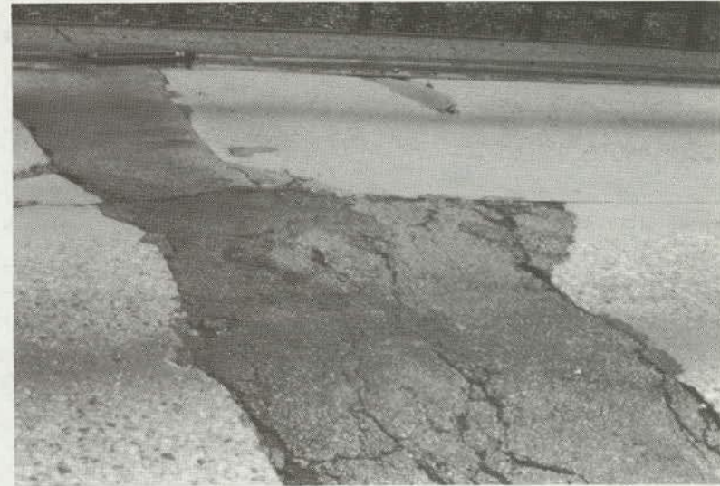
Figure 78. High-Severity Asphalt Patch Deterioration.
