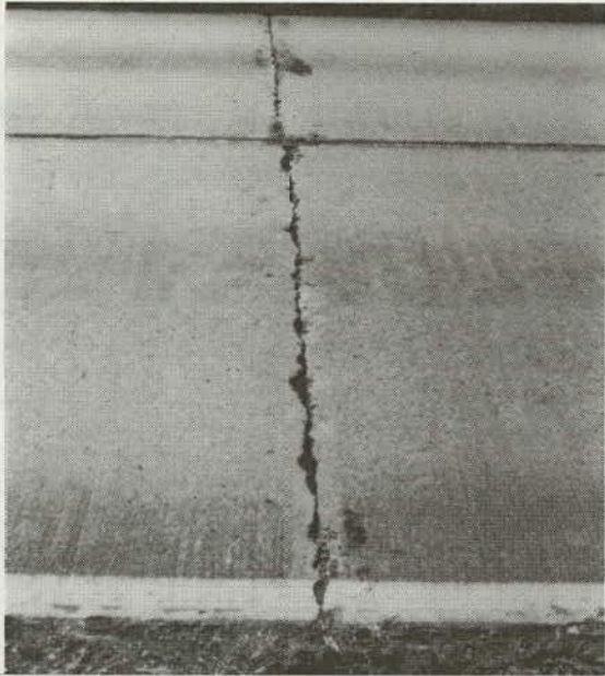
Figure 43. Low-Severity Spalling (Transverse Joint).
