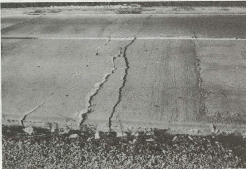
Figure 139. High-Severity Concrete Patch Deterioration.
