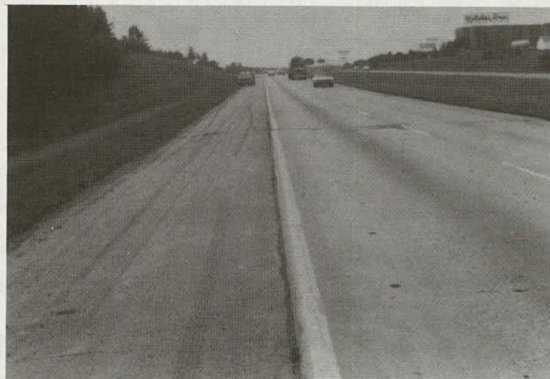
Figure 72. Lane/Shoulder Separation (Asphalt Shoulder).
