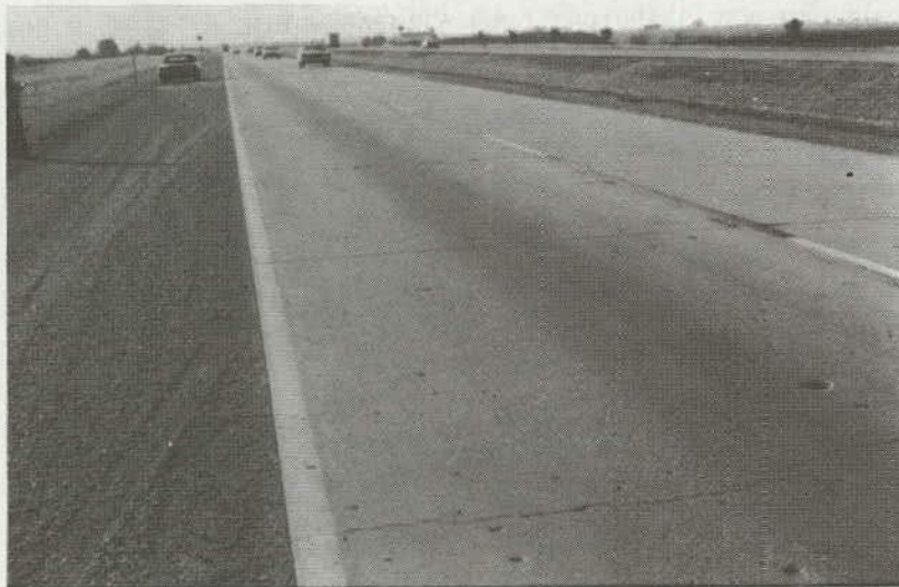
Figure 74. Lane/Shoulder Separation (high severity due to gravel shoulder).
