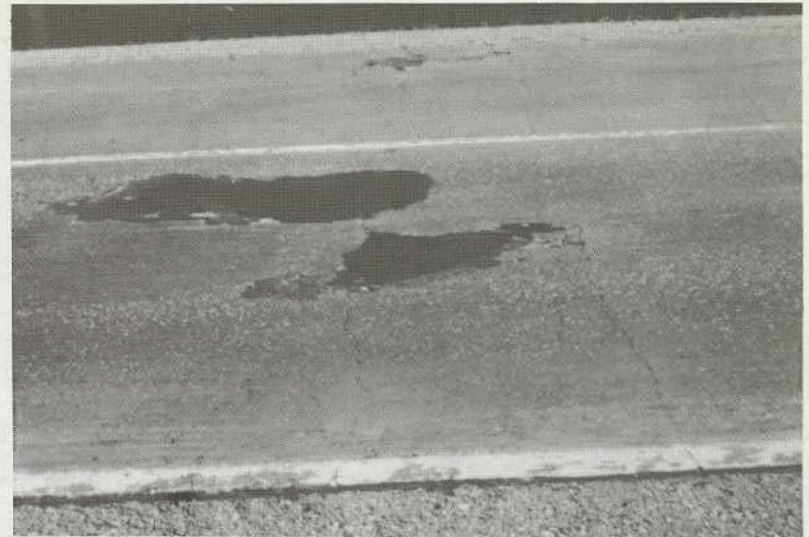
Figure 127. Medium-Severity Localized Distress.
