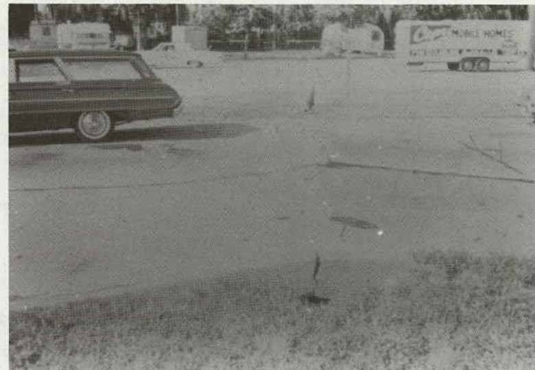
Figure 57. High-Severity Buckling Type Blow-up.
