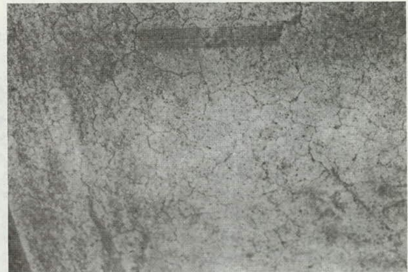
Figure 150. Low-Severity Map Cracking or Crazing.
