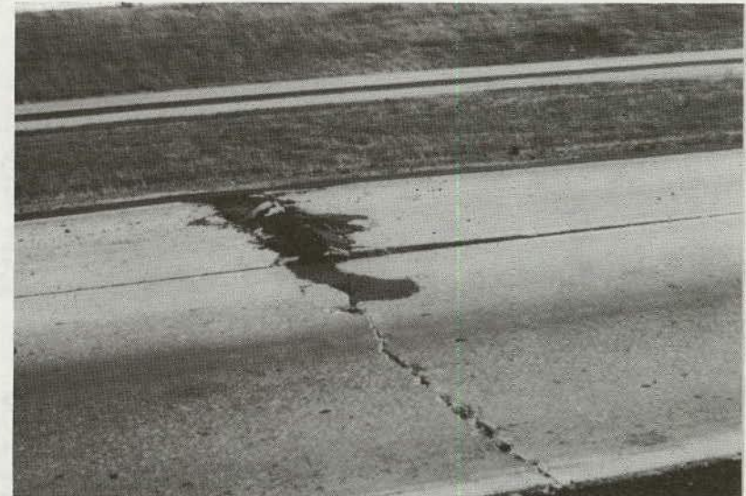
Figure 110. High-Severity Blow-up at Wide Transverse Crack.
