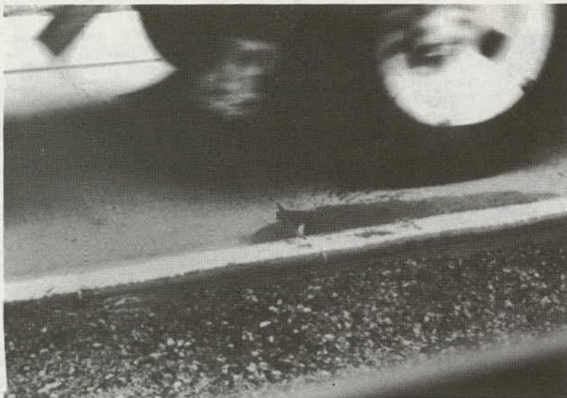
Figure 143. Low-Severity Pumping (water ejected out of transverse crack under truck wheel).
