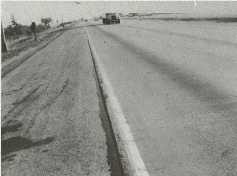
Figure 123. Medium-Severity Lane/Shoulder Joint Separation (asphalt shoulder).
