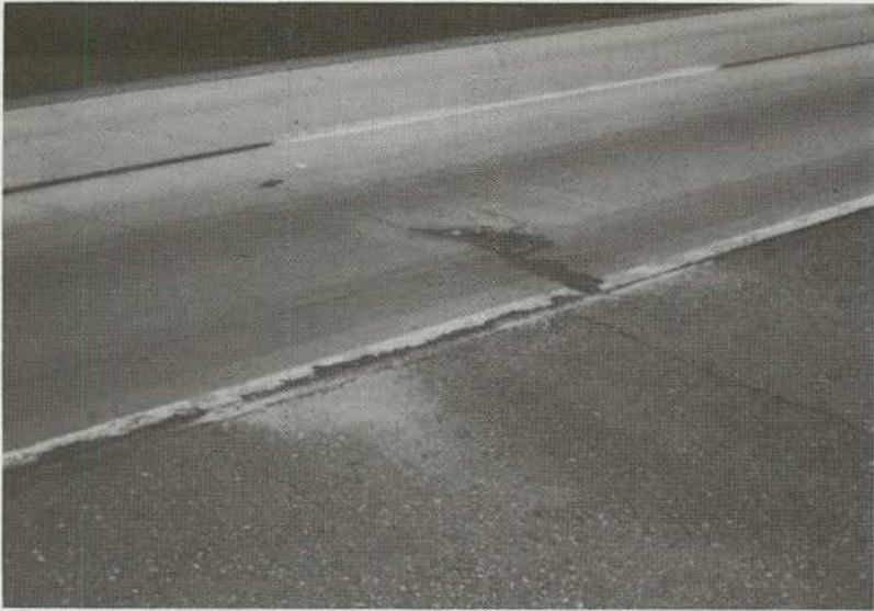
Figure 146. Medium-Severity Pumping of Fines.
