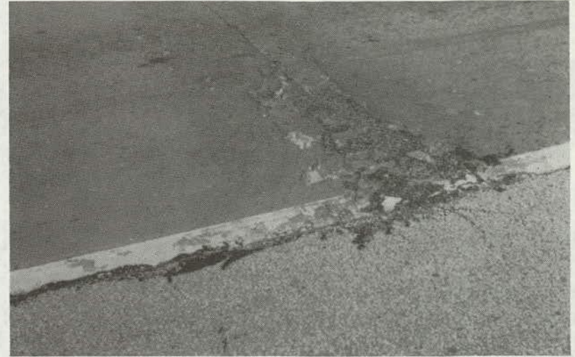
Figure 16. High-Severity "D" Cracking.
