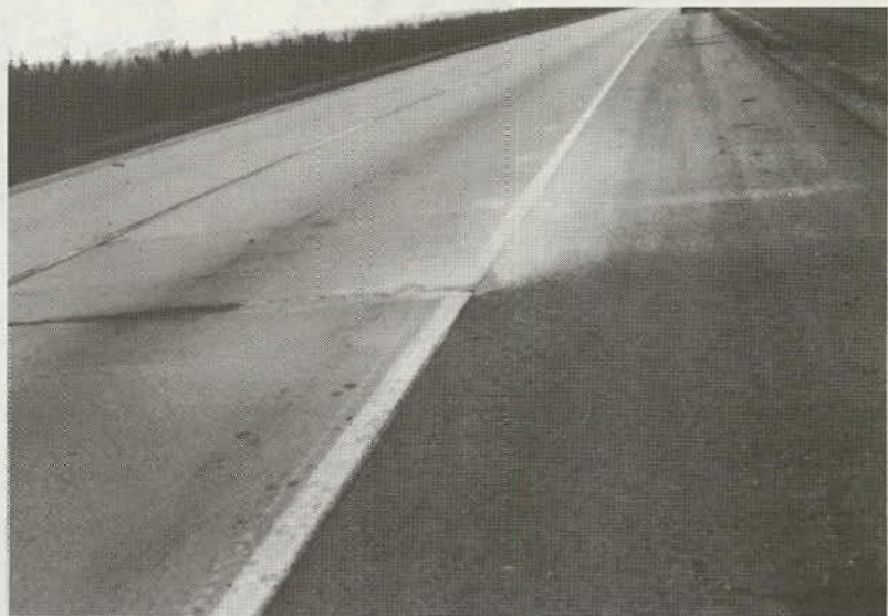
Figure 148. High-Severity Pumping of Fines.
