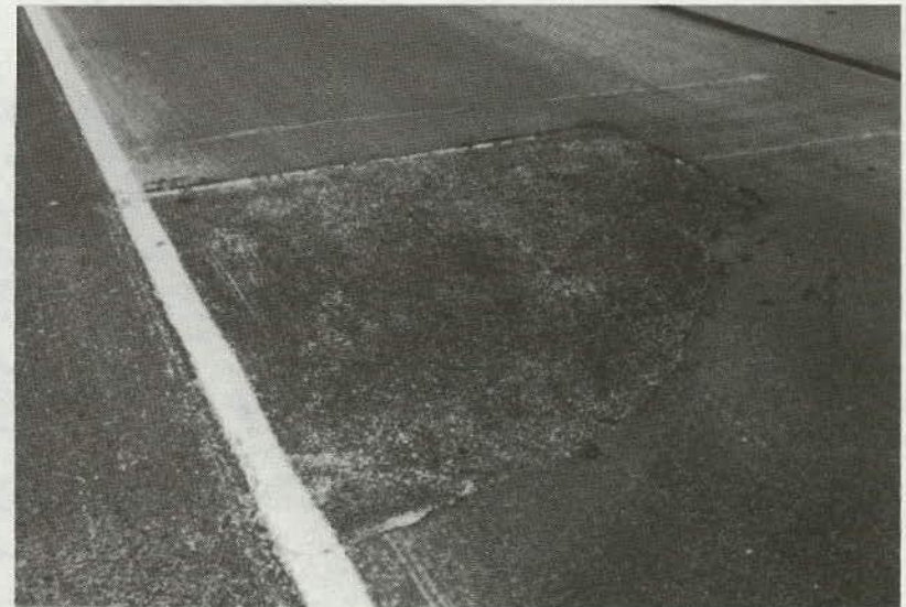
Figure 133. Low-Severity Asphalt Patch Deterioration.
