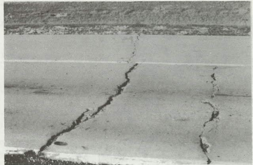
Figure 108. High-Severity Transverse Crack.
