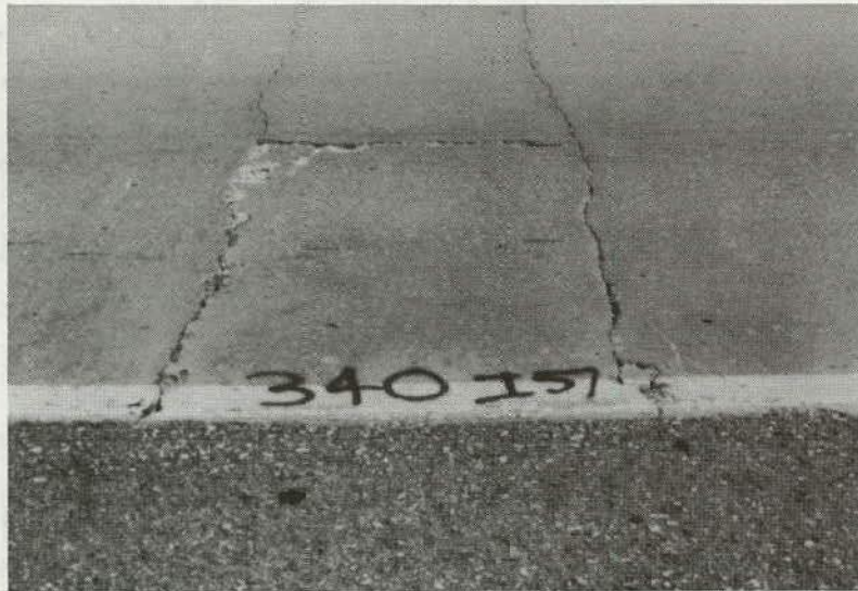
Figure 119. Medium-Severity Edge Punchout (this photo is same edge punchout as Figure 118 after one year).
