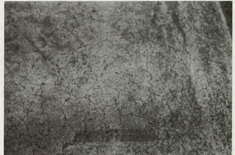
Figure 40. Map Cracking or Cracking.
