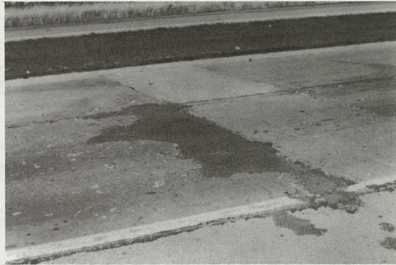
Figure 84. Patch Adjacent Slab Deterioration ("D" Cracking).
