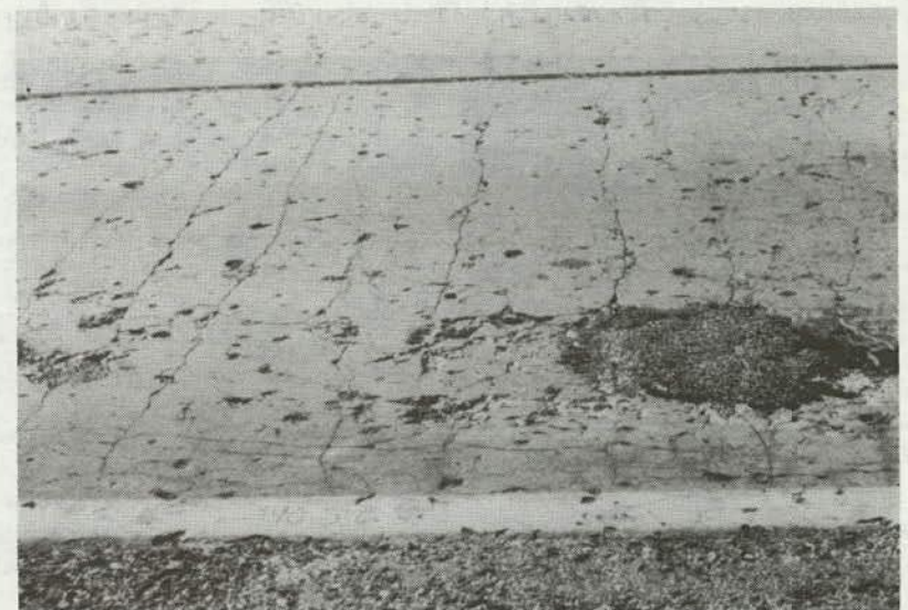
Figure 116. High-Severity "D" Cracking.
