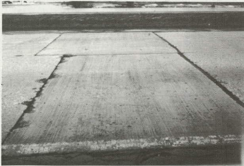
Figure 31. Medium-Severity PCC Patch Deterioration.
