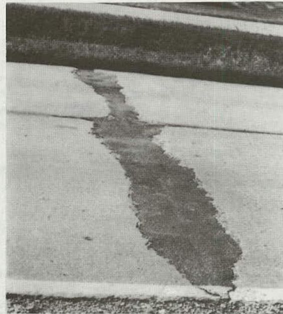
Figure 46. Medium-Severity Spalling (Transverse Joint).
