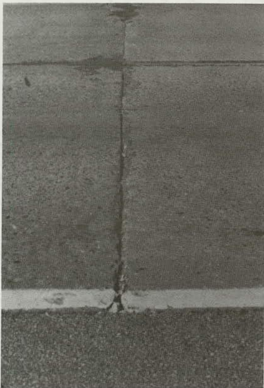
Figure 71. High-Severity Joint Seal Damage.
