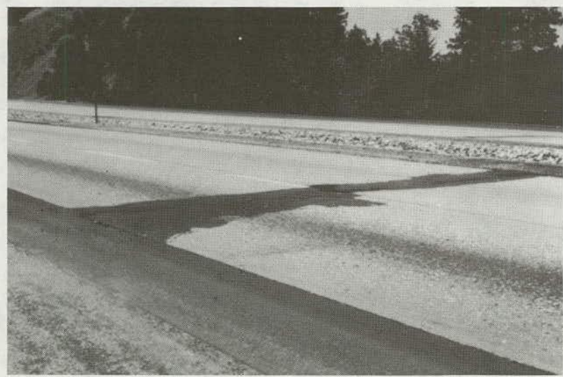
Figure 10. Medium-Severity Blow-up (temporary patch).
