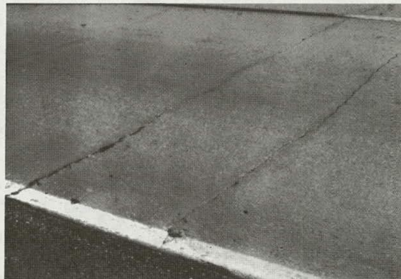
Figure 118. Low-Severity Edge Punchout (Note: a fine longitudinal crack has developed between the two closely spaced transverse cracks).
