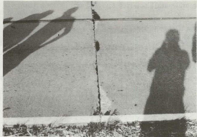
Figure 45. Medium-Severity Spalling (Transverse Joint).
