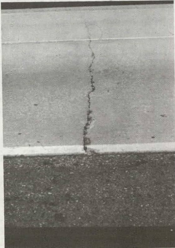
Figure 155. Medium-Severity Spalling of Transverse Cracks.
