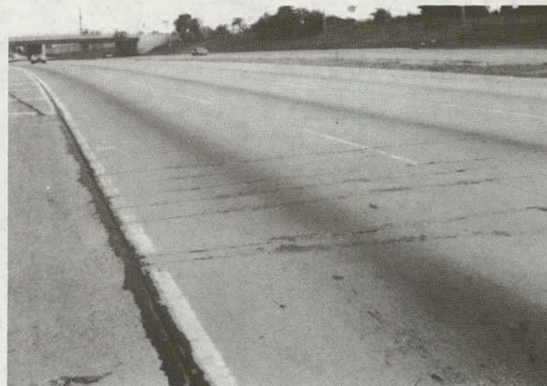
Figure 153. Low-Severity Spalling of Transverse Cracks (these cracks are tight beneath the spalled surface).
