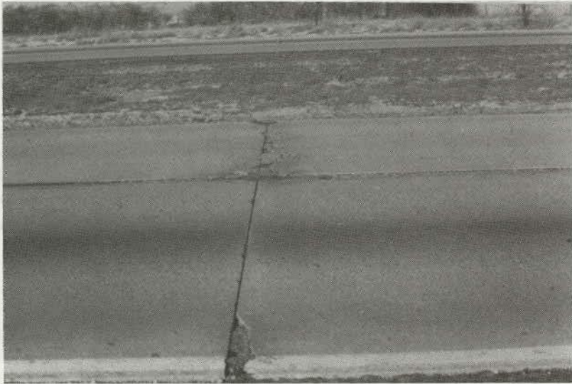
Figure 15. Medium-Severity "D" Cracking.
