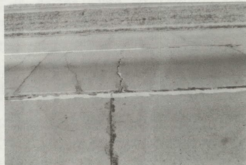
Figure 137. Medium-Severity Concrete Patch Deterioration.
