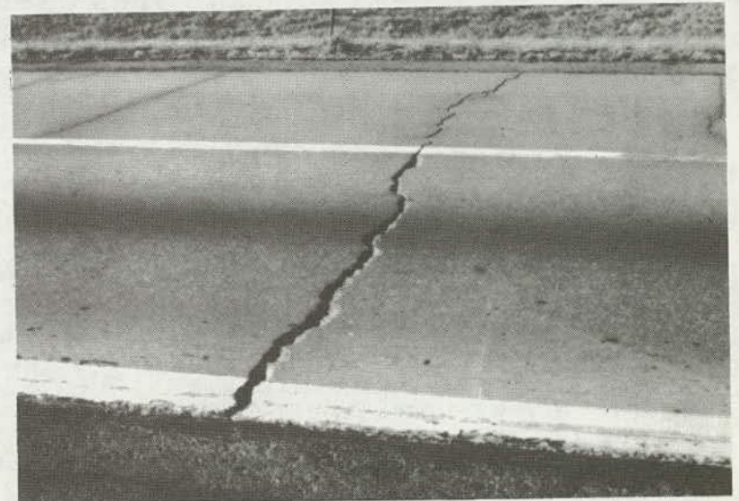
Figure 157. High Severity Spalling of Transverse Crack (Note: see Figure 112 for an example of high severity construction joint spalling).
