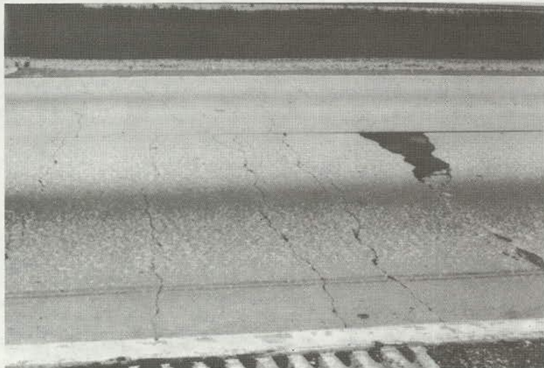
Figure 126. Medium-Severity Localized Distress.
