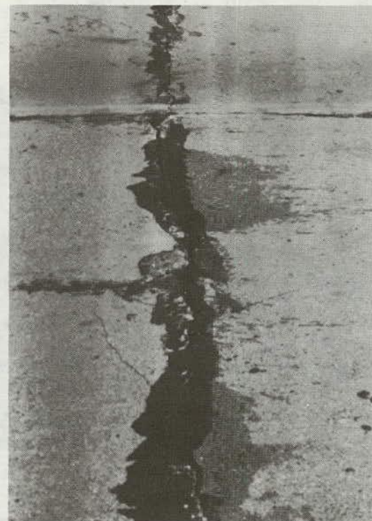
Figure 86. Low-Severity Pumping (Water Bleeding).
