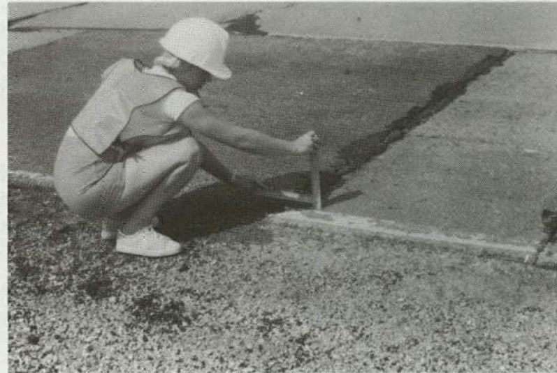
Figure 33. Medium-Severity Asphalt Patch Deterioration.
