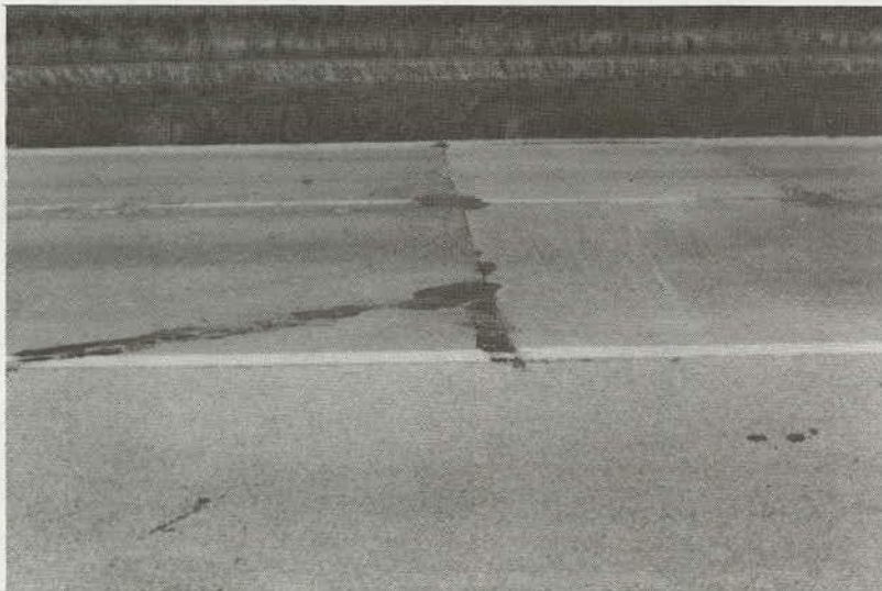
Figure 83. Patch Adjacent Slab Deterioration (Corner Break).
