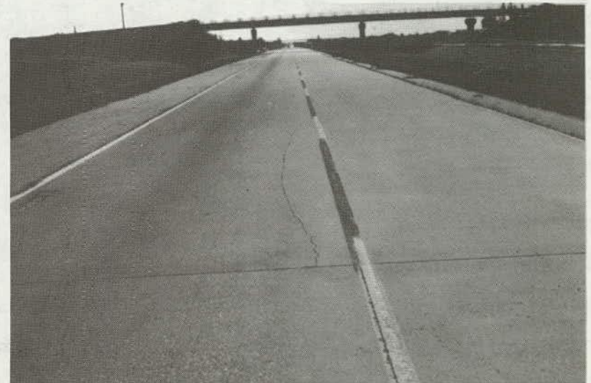
Figure 75. Low-Severity Longitudinal Crack.
