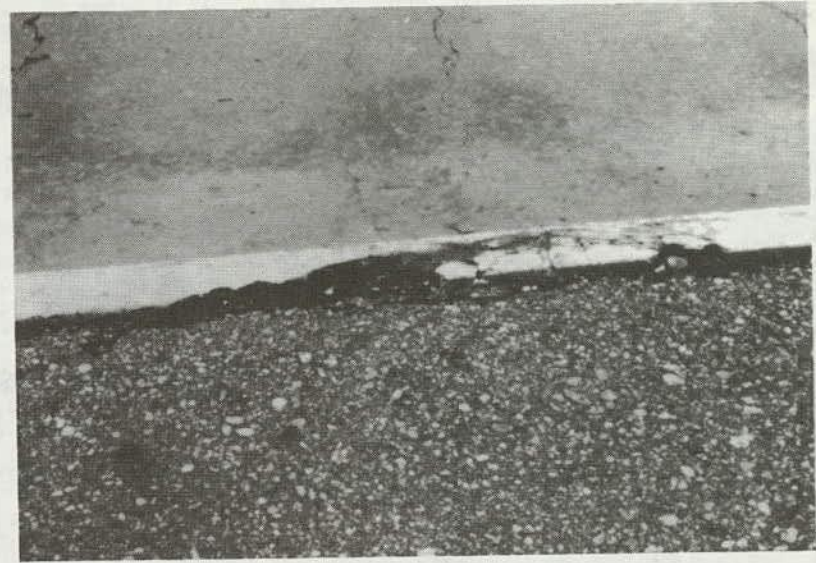
Figure 156. Medium-Severity Spalling of Longitudinal Joint.
