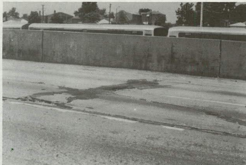
Figure 76. High-Severity Longitudinal Crack in Center Lane.
