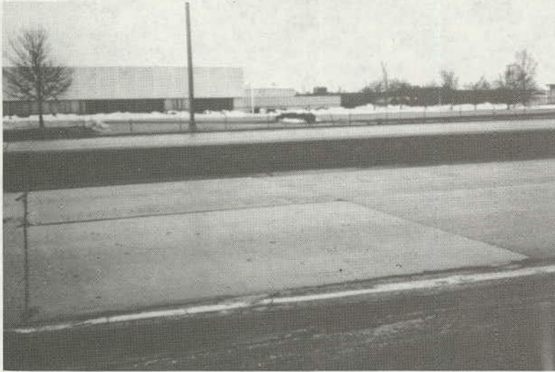
Figure 30. Low-Severity PCC Patch Deterioration.
