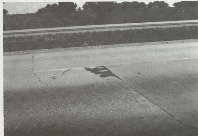
Figure 140. Patch Adjacent Slab Deterioration (spalling).
