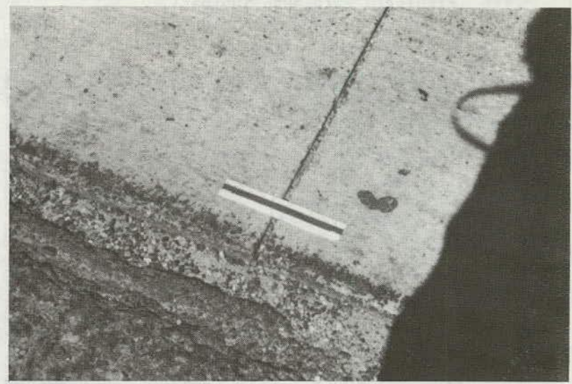
Figure 24. High-Severity Lane / Shoulder Separation.
