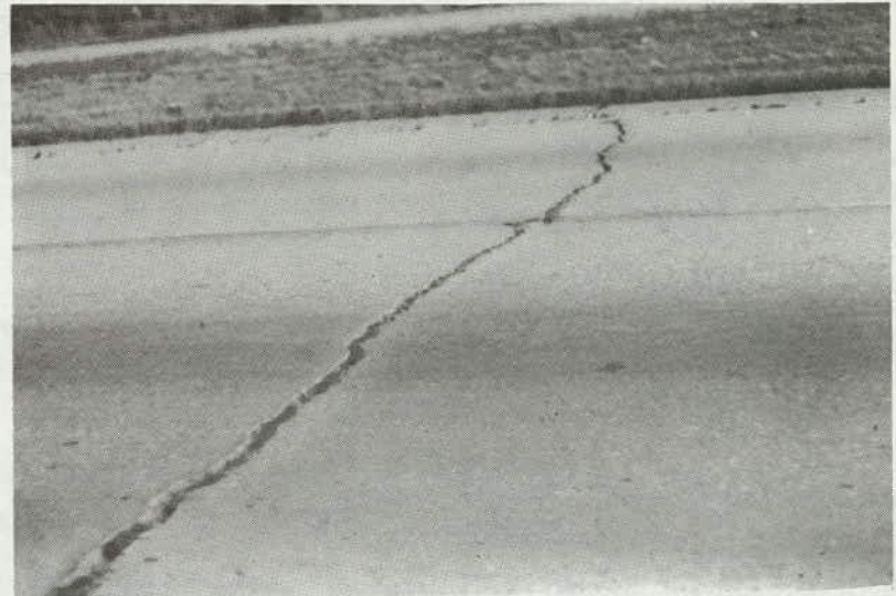
Figure 107. High-Severity Transverse Crack.
