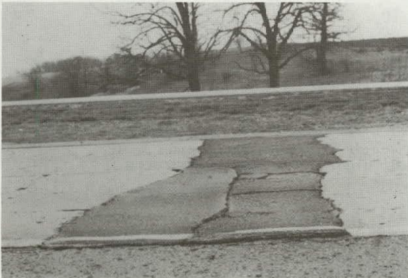
Figure 135. High-Severity Asphalt Patch Deterioration.
