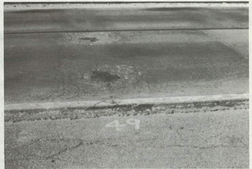
Figure 115. Medium-Severity "D" Cracking.
