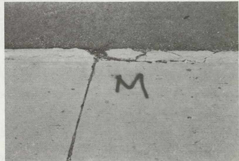
Figure 70. Medium-Severity Joint Seal Damage.
