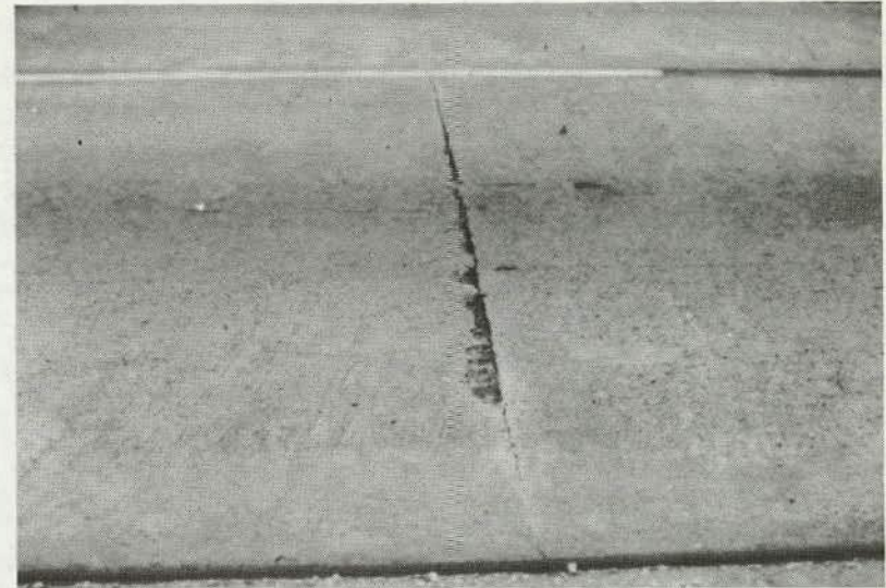
Figure 92. Low-Severity Spalling (Fray).
