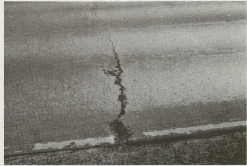
Figure 106. Medium-Severity Transverse Crack.
