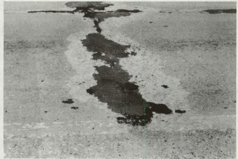
Figure 39. Scaling Near Transverse Joint.
