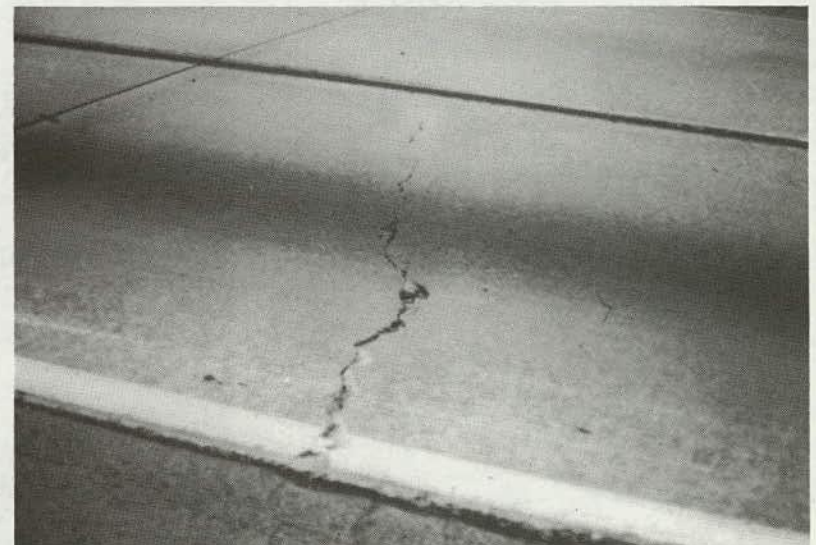
Figure 54. Medium-Severity Transverse Crack.
