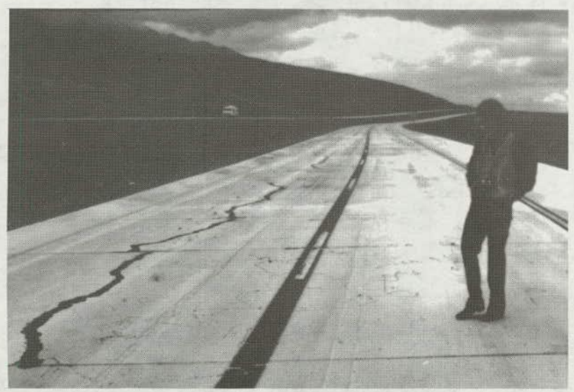
Figure 50. Swell due to Frost Heave (observe cracking).
