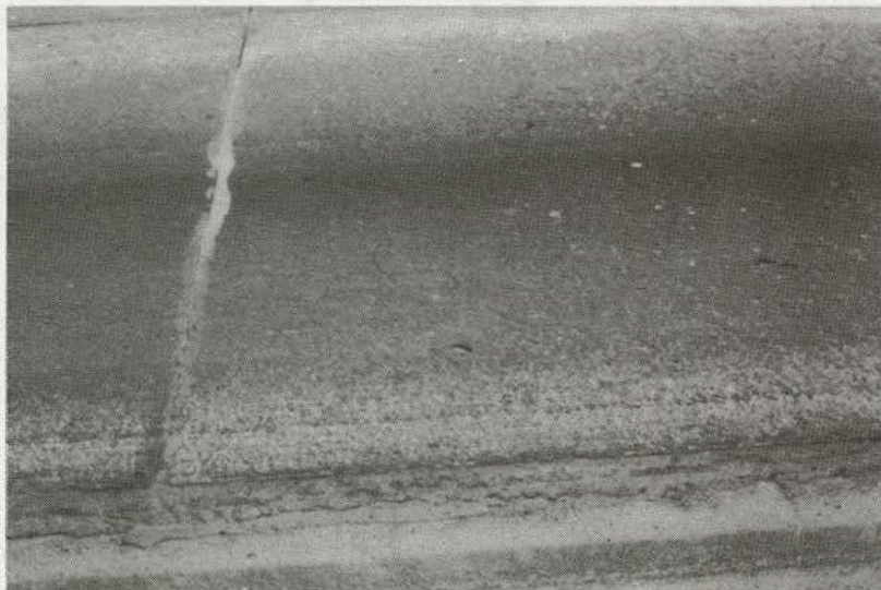
Figure 20. Low-Severity Joint Sealant Damage.
