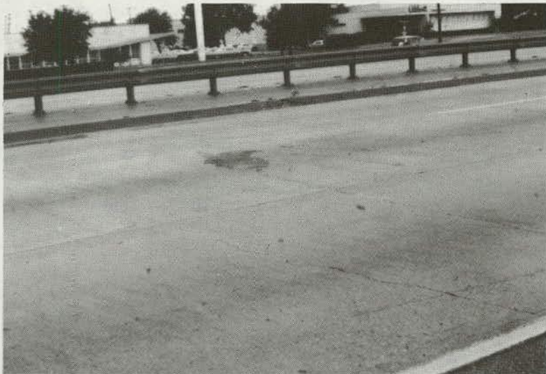
Figure 129. Medium-Severity Localized Distress.
