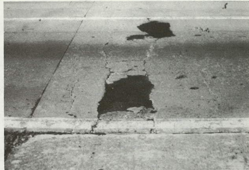
Figure 111. High-Severity Construction Joint Deterioration.
