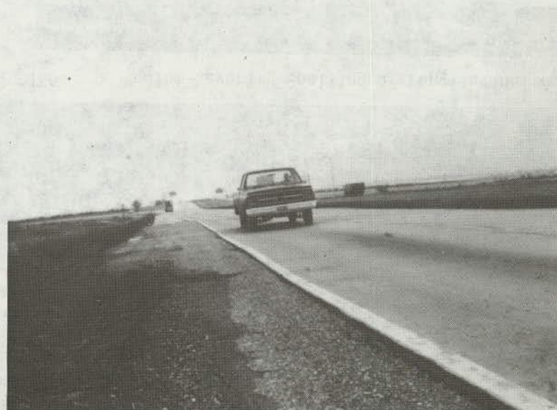
Figure 159. Swell Caused by Frost Heave (located behind truck)
