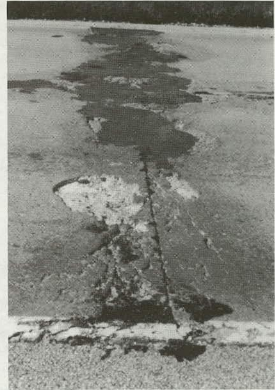
Figure 66. High-Severity "D" Cracking.
