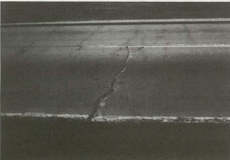
Figure 165. High-Severity Transverse Crack.
