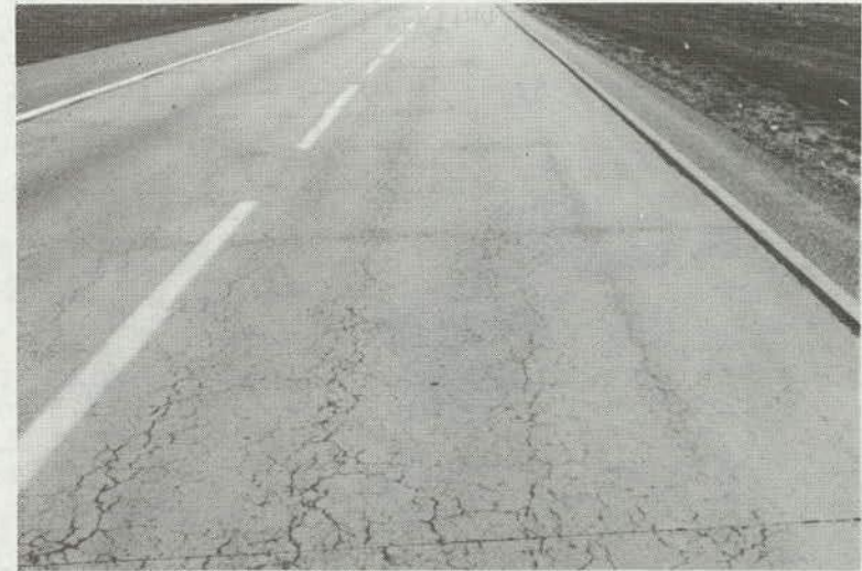
Figure 37. Medium-Severity Reactive Aggregate Distress.
