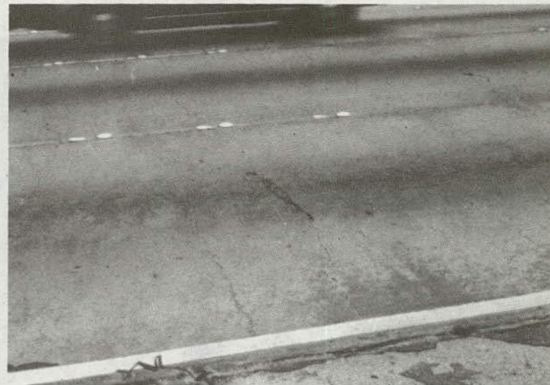
Figure 152. Low-Severity Spalling of Transverse Cracks.
