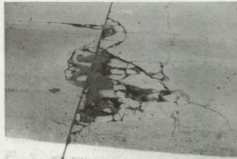
Figure 112. High-Severity Construction Joint Deterioration.
