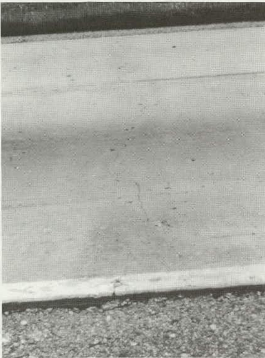
Figure 114. Low-Severity "D" Cracking.
