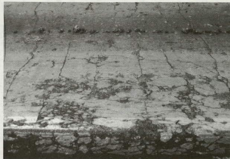
Figure 117. High-Severity "D" Cracking (note exposed edge of slab at bottom of photo).
