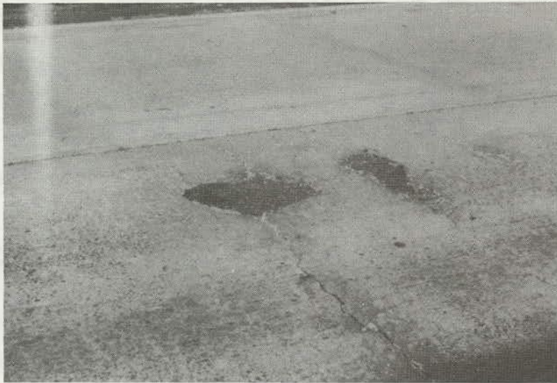
Figure 125. Medium-Severity Localized Distress.
