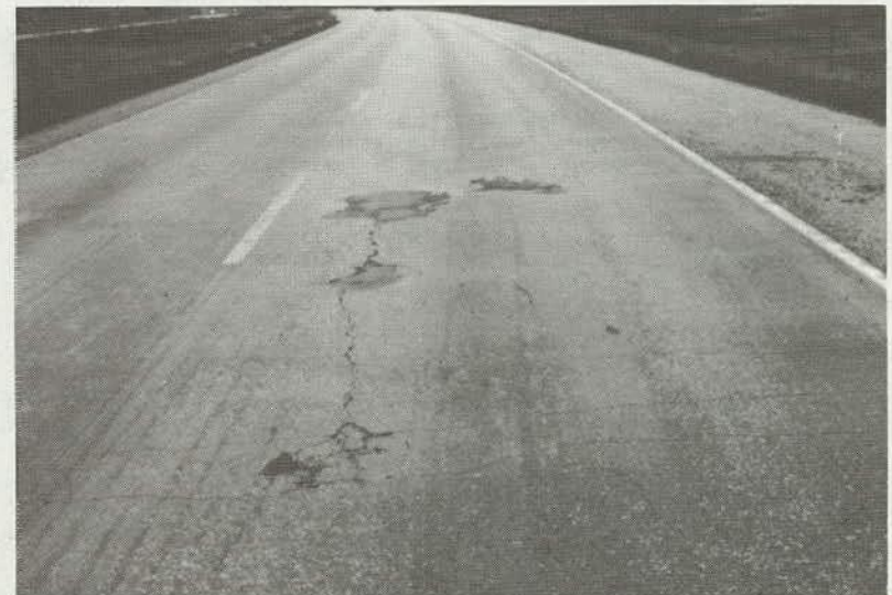
Figure 128. Medium-Severity Localized Distress.
