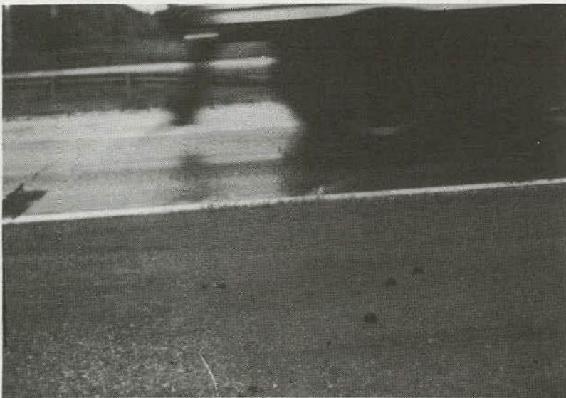
Figure 144. Low-Severity Pumping (water ejected out of longitudinal joint under truck wheel).
