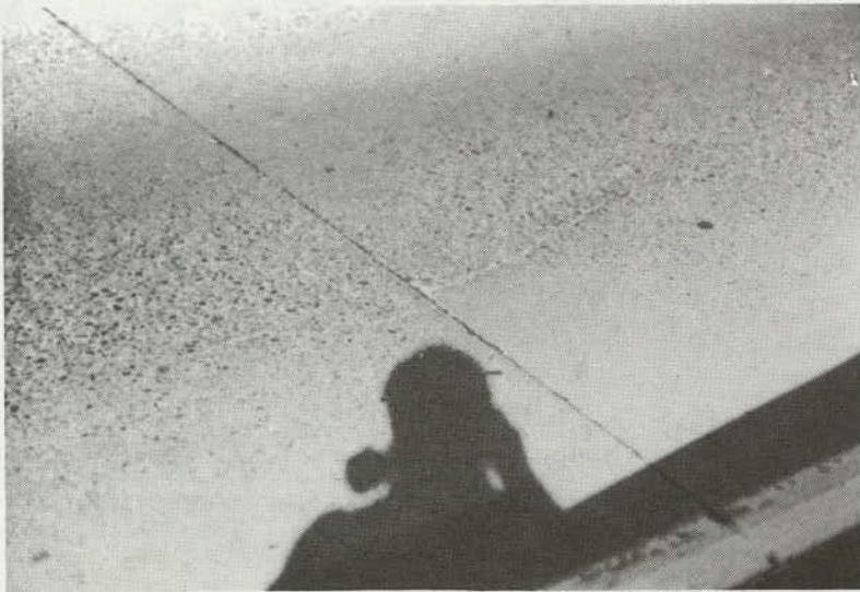
Figure 26. Low-Severity Longitudinal Crack.
