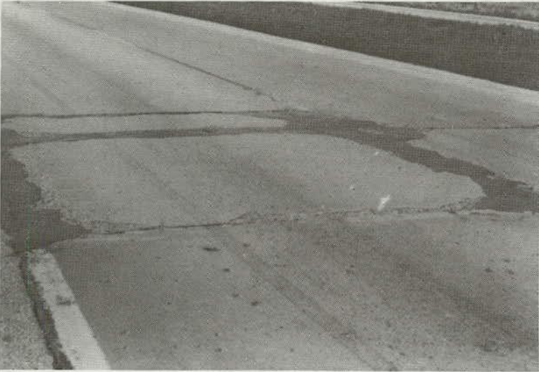
Figure 80. Medium-Severity Concrete Patch Deterioration.
