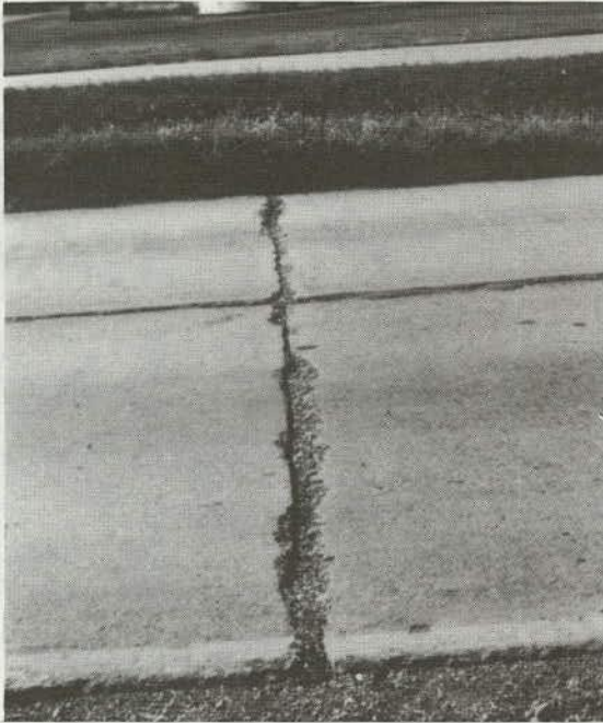
Figure 47. High-Severity Spalling (Transverse Joint).
