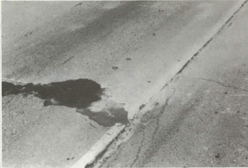
Figure 87. Medium-Severity Pumping (pumped material like this occurs only at a few of the joints and cracks).
