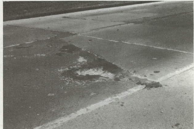
Figure 85. Patch Adjacent Slab Deterioration (Spalling and "D" Cracking).
