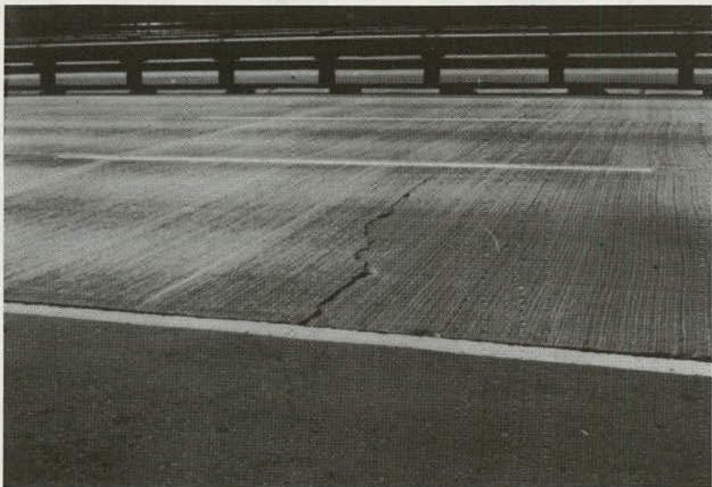
Figure 55. Medium-Severity Transverse Crack.
