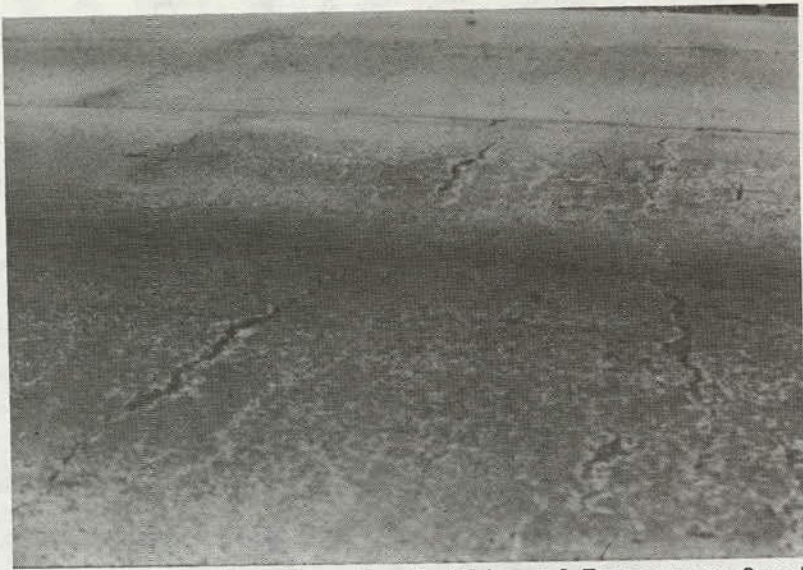
Figure 154. Low-Severity Spalling of Transverse Cracks.
