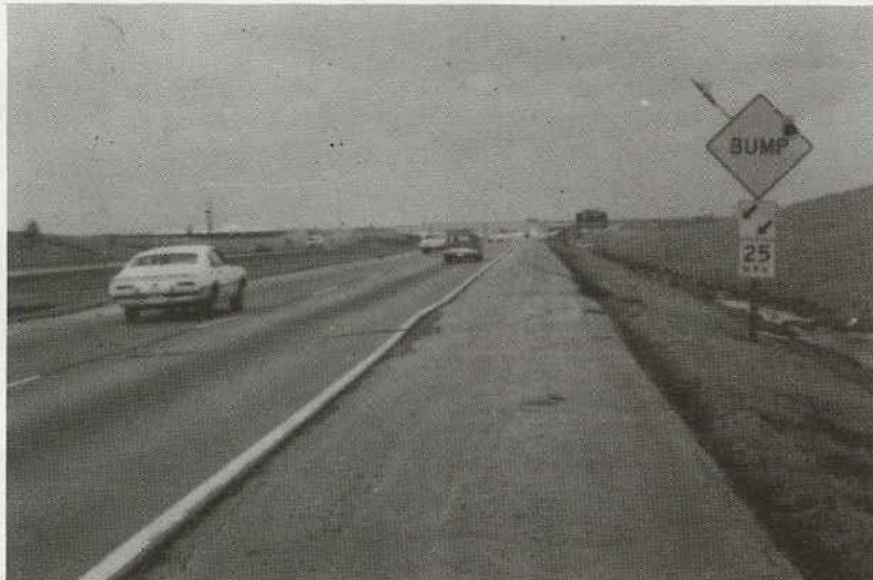
Figure 102. Swell Due to Frost Heave.
