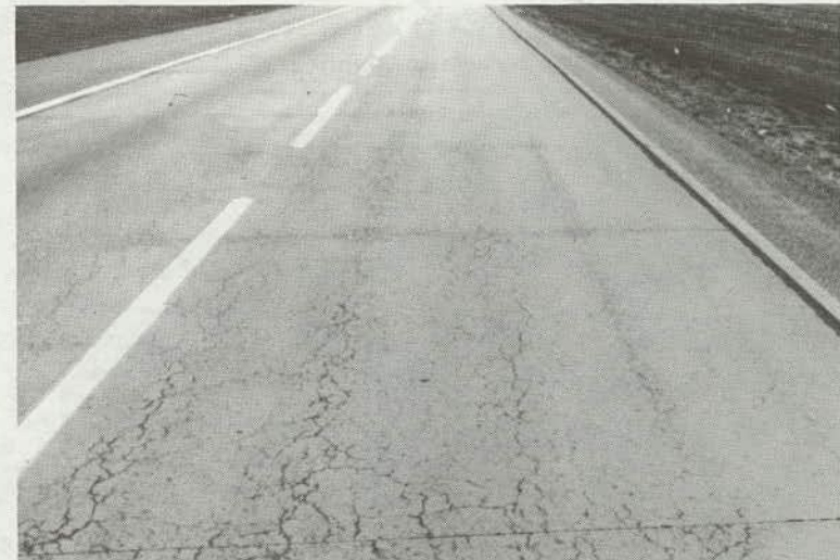
Figure 89. Medium-Severity Reactive Aggregate Distress (Photo for Jointed Plain Concrete Pavement).
