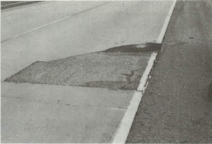
Figure 134. Medium-Severity Asphalt Patch Deterioration (same patch as Figure 133 after 2 years).
