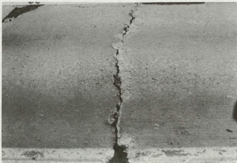
Figure 56. High-Severity Transverse Crack.
