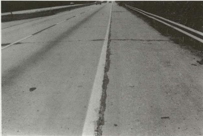
Figure 73. Lane/Shoulder Separation (PCC Shoulder).
