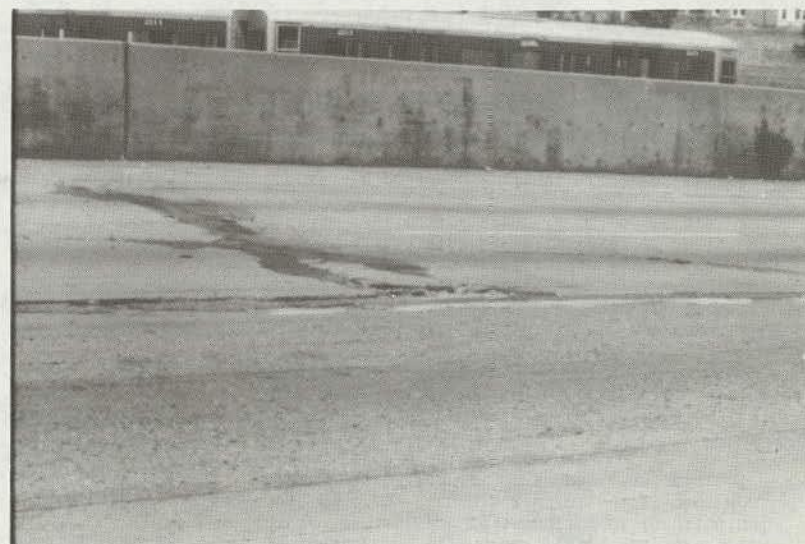
Figure 77. Longitudinal Joint Faulting.
