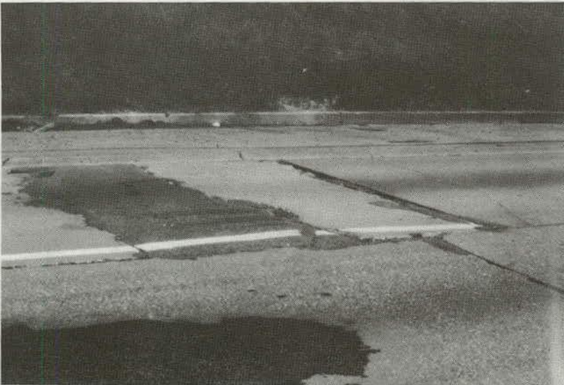
Figure 81. High-Severity Concrete Patch Deterioration.
