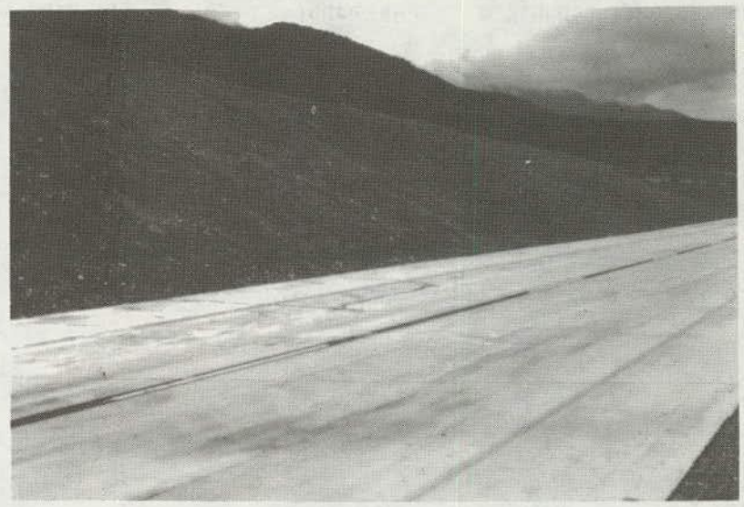
Figure 51. Swell Due to Frost Heave (observe cracking of slab).
