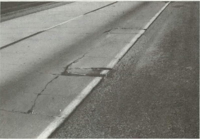
Figure 147. Medium-Severity Pumping of Fines.
