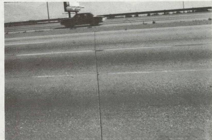
Figure 22. High-Severity Joint Sealant Damage (sealant generally missing).
