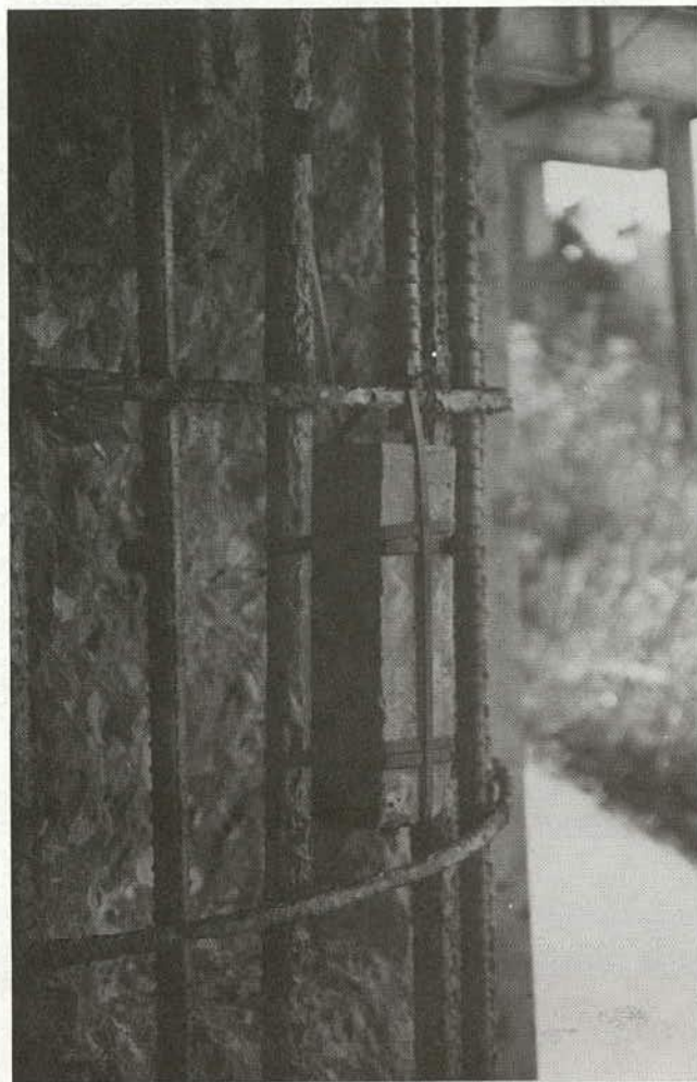
Figure C-8. Precast maroccell assembly suspended between reinforcing bars with plastic ties prior to casting repair concrete.
