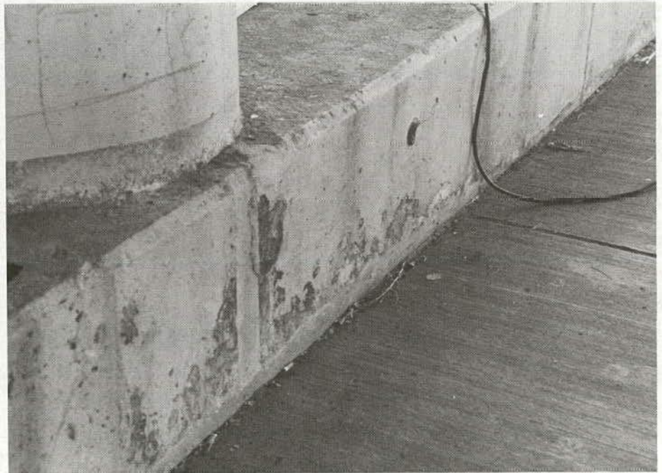
Figure E-3. Scaled coating on the side of the base.
