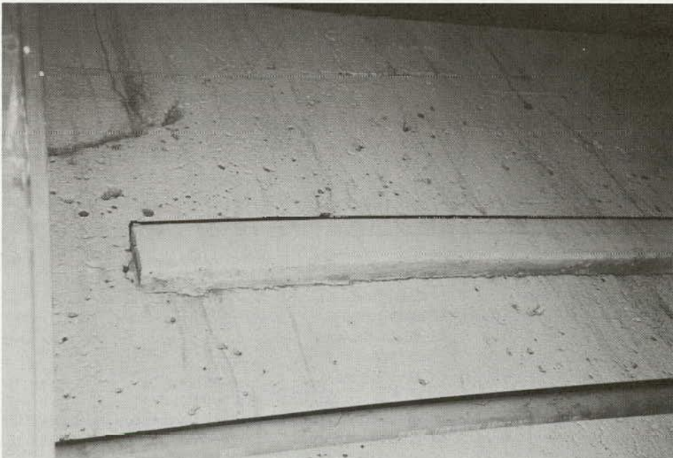
Figure E-1. Loss of bond between the concrete and the precast anode.
