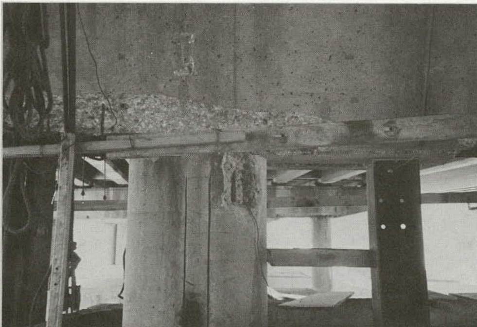
Figure C-7. Ground wire attached to exposed reinforcing bar of column.
