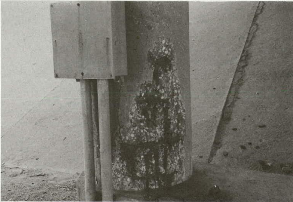
Figure C-3. Deteriorated base of north column.
