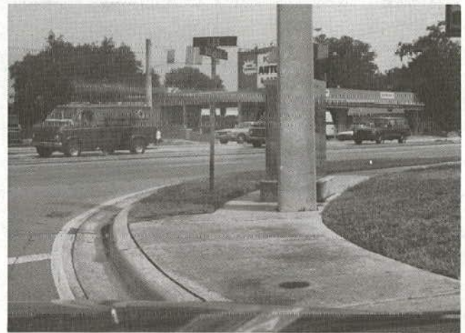
Figure 8. Major obstacles unnecessarily placed in sidewalk.
