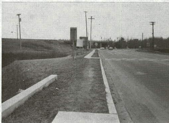
Sidewalk entering the area from U.S. 50 with crossing of Garden City Drive. Note worn path after the sidewalk ends.
