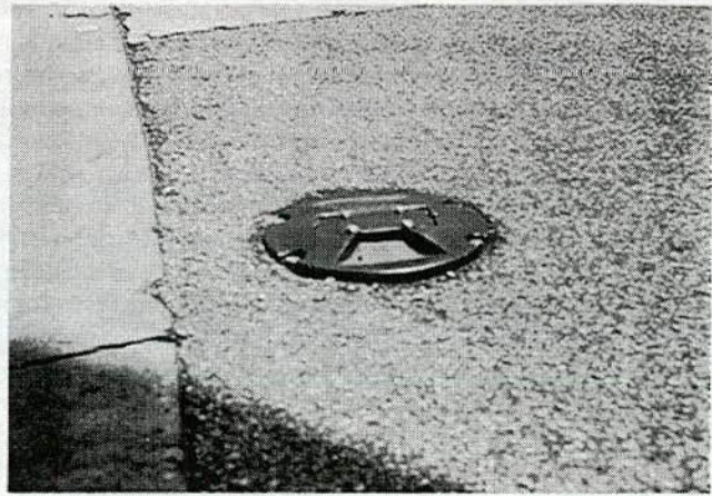
Figure 84. Embedded pavement marking lights.
