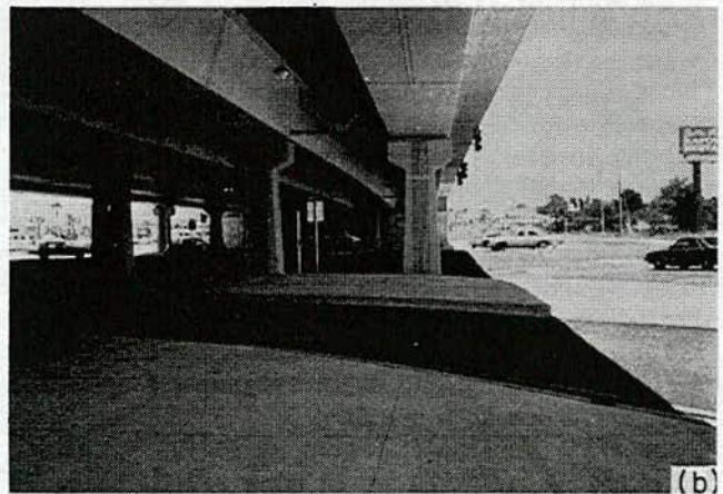
Figure 87. Lighting design underneath the overpassing bridge: (a) lighting units attached to mainline girders; (b) lighting units attached to bridge deck.
