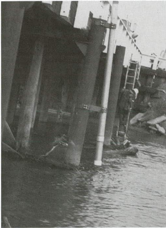
Figure 47. Sonic device support installation at State Highway 144 bridge near Orchard, CO (CO1).
