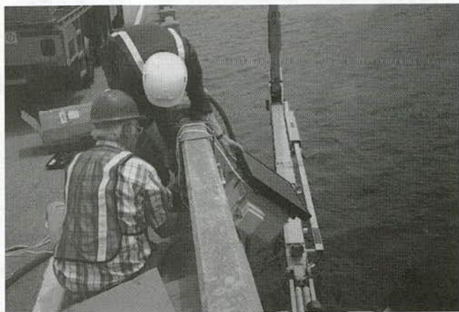
Figure 31. Nassau Sound sliding collar—datalogger housing and solar panel (Site FL2).
