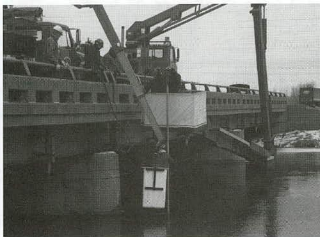
Figure 32. Installation of magnetic sliding collar device at Muskegon River bridge (Site M11).
