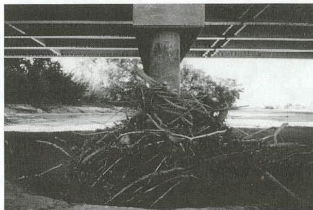
Figure 56. Debris and scour hole “in the dry” on San Antonio bridge pier on Rio Grande, NM (Site NM2).
