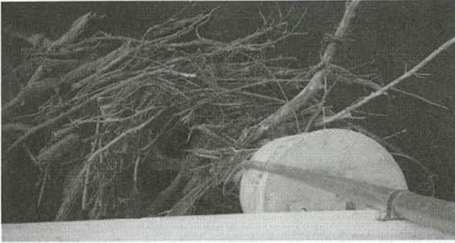
Figure 42. Debris accumulation on sliding collar device at Minnesota bridge no. 23015 (Site MN2).
