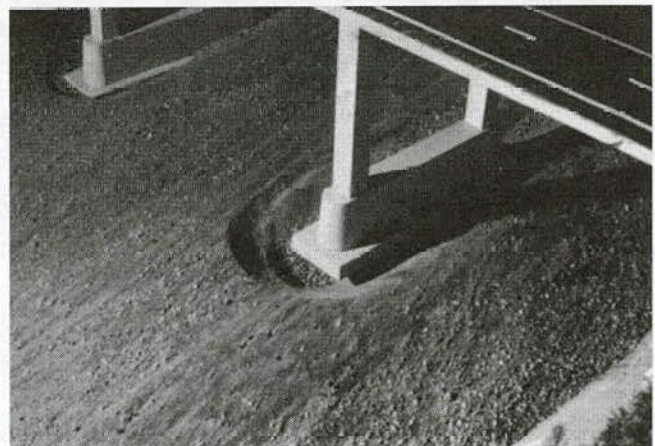
Figure 74. Schoharie Creek Pier 3 from the right bank showing the scour hole in the dry channel for 1987 flood conditions.
