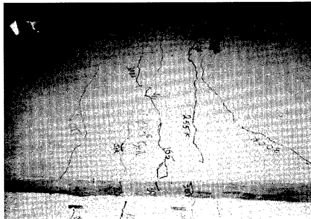
Figure 16. Cracks on top surface over the girder line.
