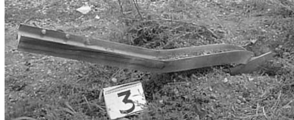
Figure 53. Bent Steel Weak Guardrail Post
