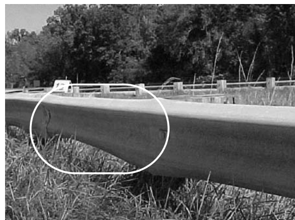
Figure 70. Deformation of W-beam guardrail.
