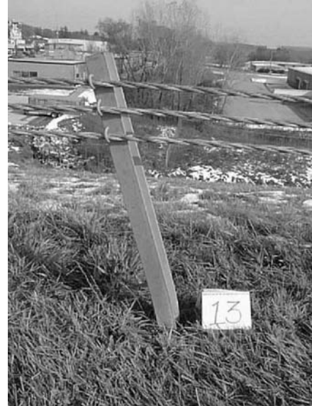
Figure 68. Bent post (cable guardrail)
