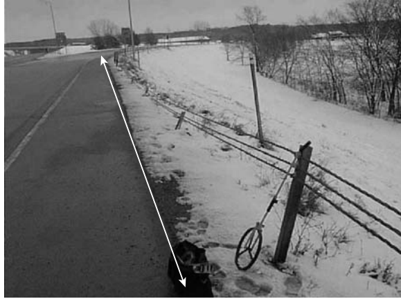
Figure 57. Damaged Length of Guardrail
