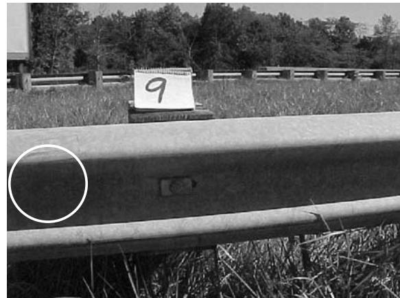
Figure 69. Marks on W-beam guardrail.
