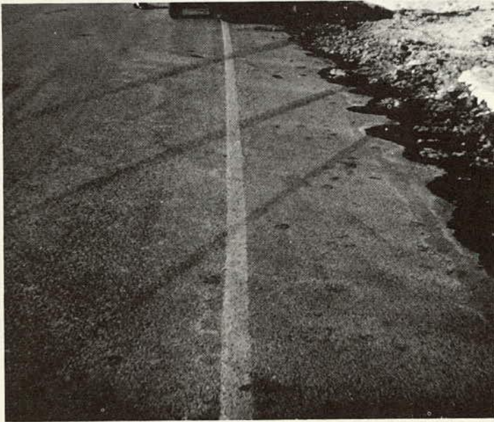
SKID MARKS LEFT BY VEHICLE AT EDGE OF PAVEMENT
