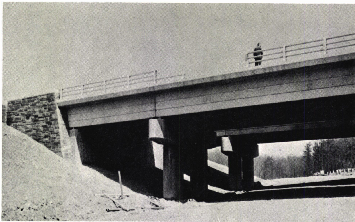
Figure 2. Example of railing penetration.
