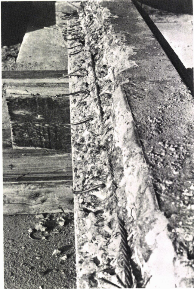
Figure H-3. Appearance of steel strand after chipping away concrete cover.
