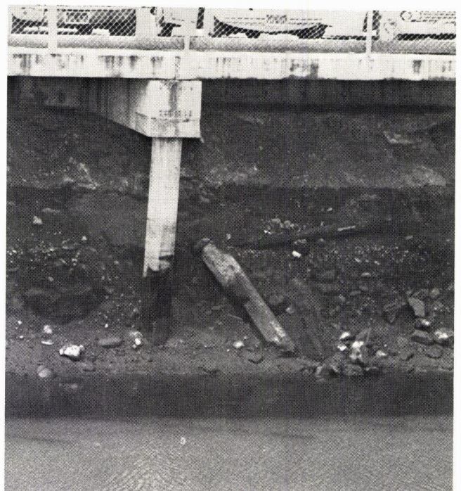
Figure H-2. Exposure site of 10-ft pretensioned pile section on Petaluma River bank, California.
