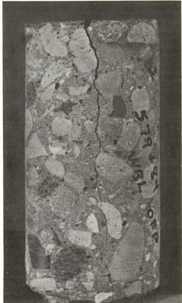
Figure 3. Pavement core through crack.
