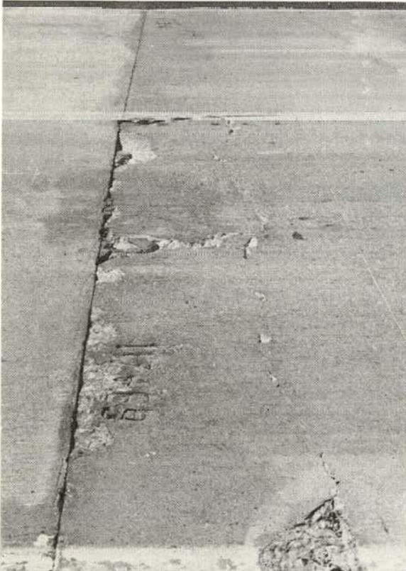
Figure 12. Construction joint failure caused by lack of consolidation.
