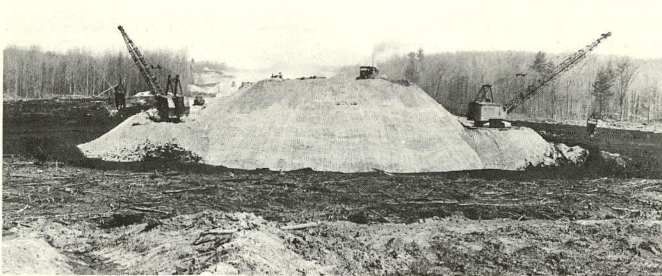
Figure 6(a). Marsh displacement (45 ft deep) and embankment construction to surcharge grade (Michigan).
