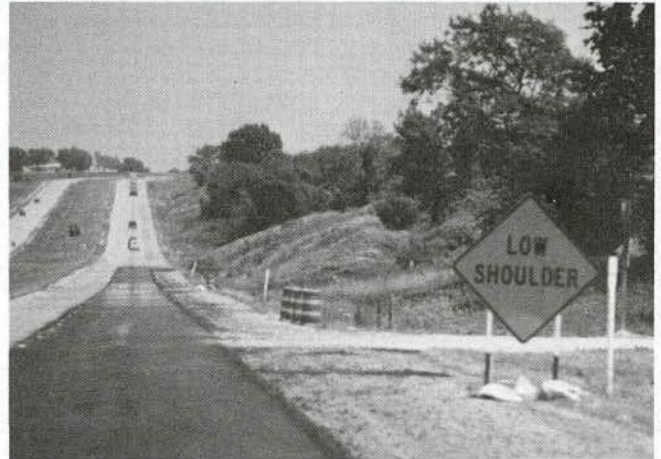
FIGURE 1 Dropoff and warning sign.
