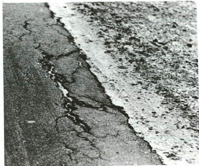
FIGURE A-5 Flexible pavement edge cracking (15).
