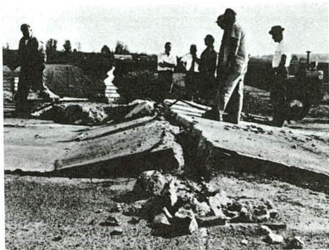
FIGURE A-8 Blowup of portland cement concrete pavement (15).
