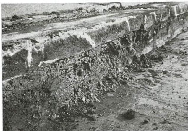
FIGURE 4 Examples of inadequate drainage: (a) water bleeding up through cracks in pavement; (b) base failure caused by contamination of aggregate with fines.
