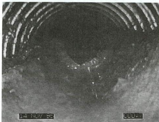
FIGURE 14 Problems identified by video camera inspection of edgedrains (49): (a) rodents' nest; (b) heavily silted drains.
