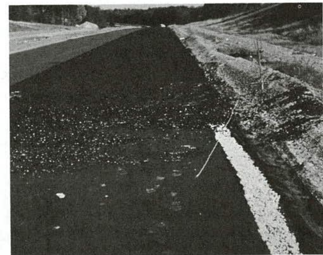
FIGURE 13 Permeable base construction; (a) placement using an asphalt spreader box; (b) closeup of in-place permeable base; (c) asphalt stabilized permeable base placed over a geotextile separator and the edgeline.
