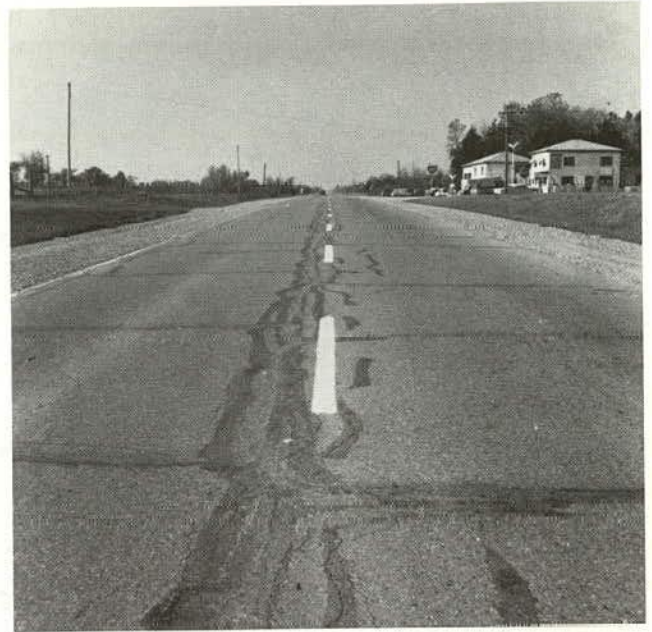
Figure 11. Pavement in Ontario severely affected by low-temperature contraction cracks (25).
