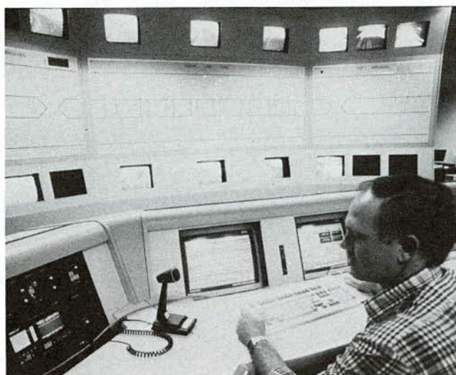
FIGURE 5 Glenwood Canyon Tunnel TMC control room with operator.
