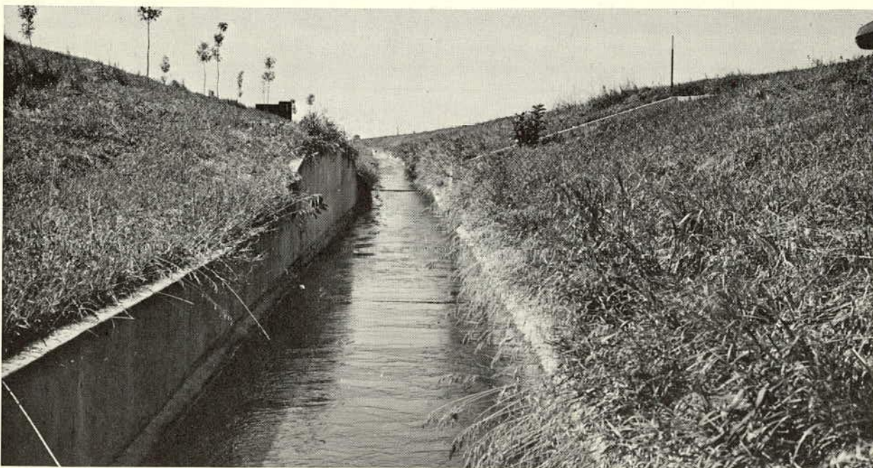
Figure 38. This paved channel is a traffic hazard when located near the roadway.
