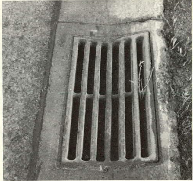
Figure 33. Drainage inlet designed for use with low mountable curb. Bars are oriented in the direction of flow.
