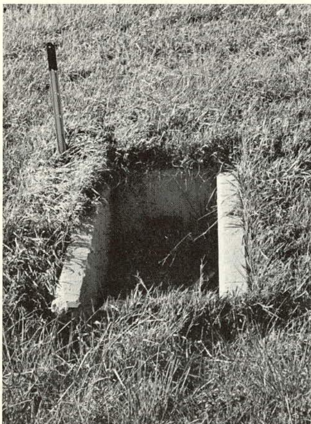
Figure 20. U-type culvert end section is dangerous when located within the recovery area. Post marker warns traffic and maintenance workers.
