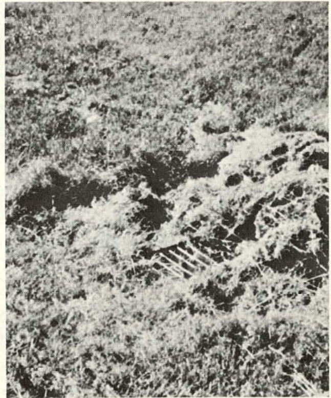
Figure 9. Capacity of drop inlet is threatened by debris and overgrowth.
