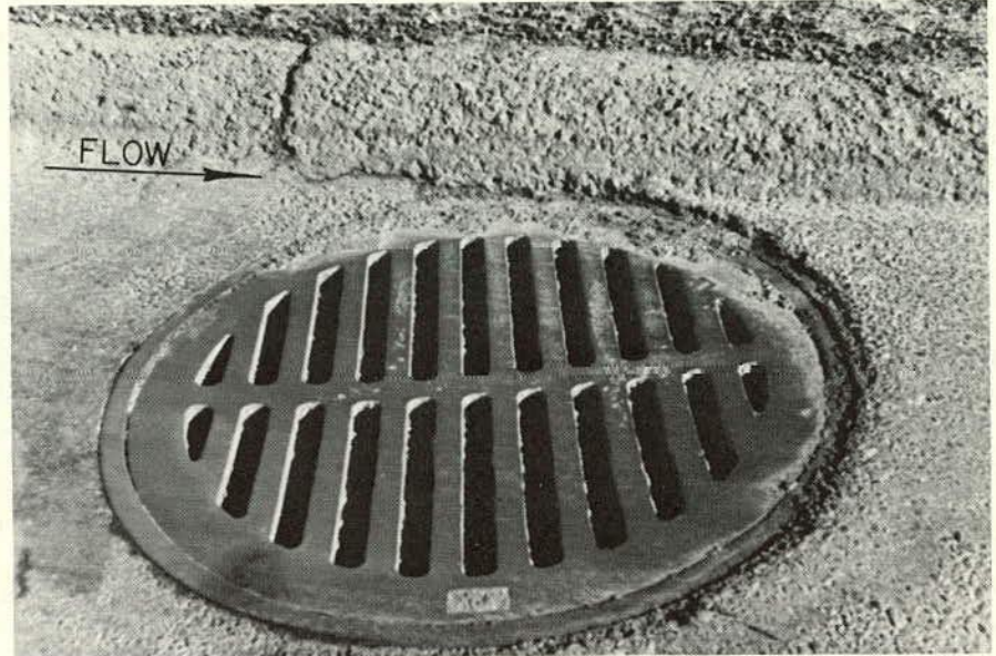
Figure 35. Improper grate orientation, reducing inlet capacity.
