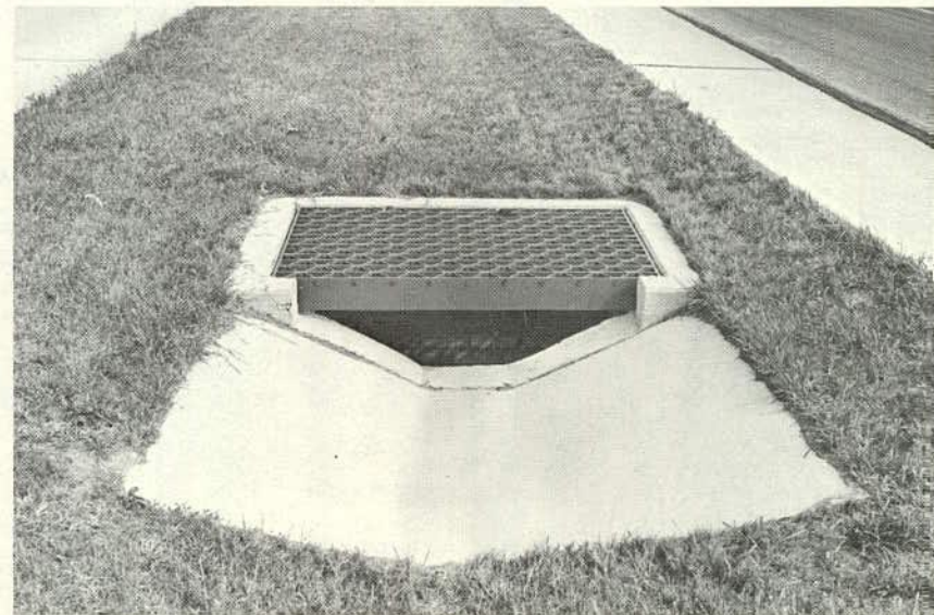
Figure 13. Drop inlet (in median) with exposed vertical face where flow enters the structure.
