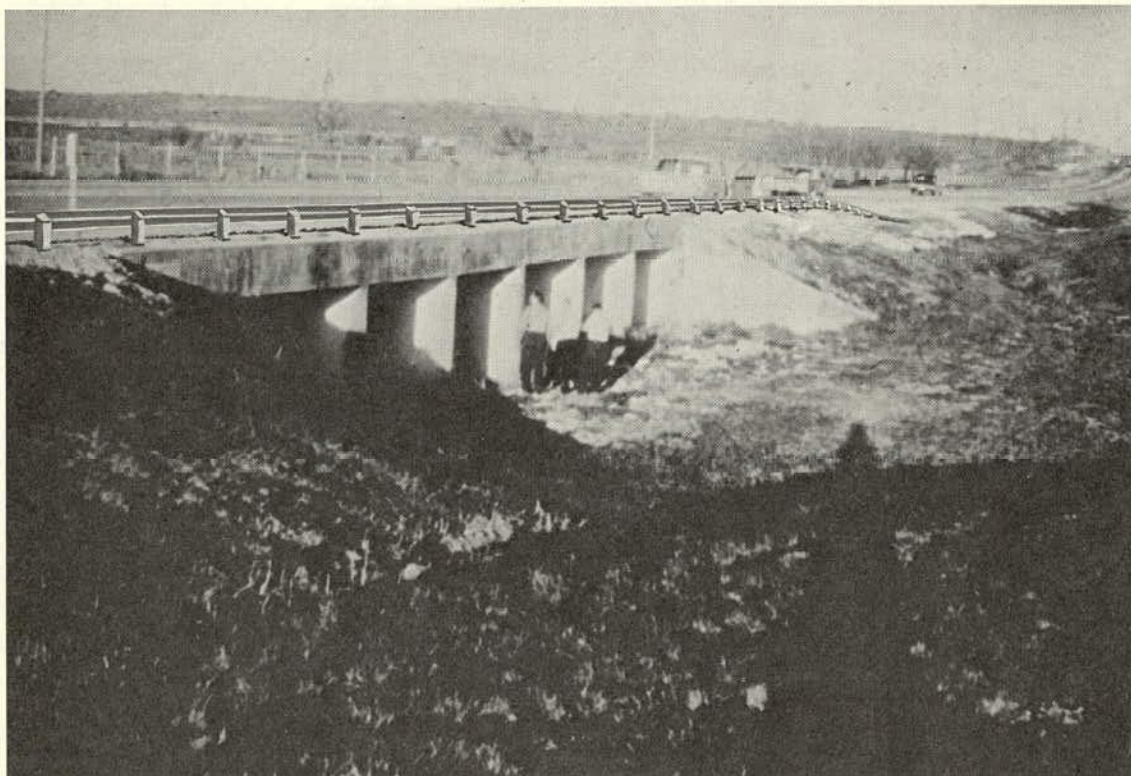
Figure 29. A dangerous situation without recovery area or protection (top). Guardrail installation is the least expensive method of affording some protection to traffic (bottom).
