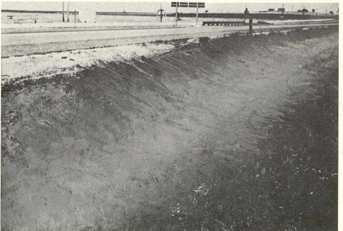
Figure 28. Closing of median crossover or drive entrance with guardrail barrier compounds hazards (top). Preferred solution would be to remove both the drainage structure and the guardrail and regrade the slope (bottom).
