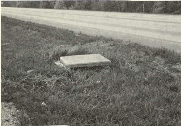
Figure 14. A concrete inlet cover weighing more than 750 lb that has been displaced by vehicle impact.
